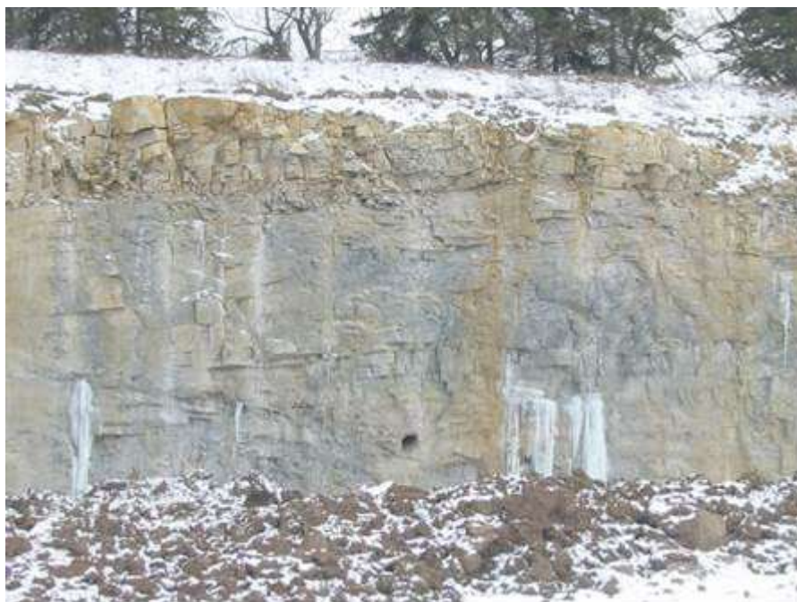
Figure 3. A hydrologically-inactive large void near the base of the south-east face of the quarry, together with ice build-ups indicating much smaller channels that are active and discharge water.
