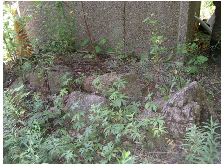
Photo 6 – Side view of typical Control Valve (CV) Hut. GEC 2017-08-25
