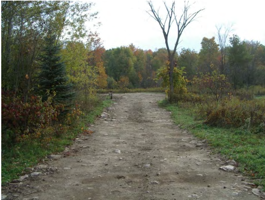
Photo 7 – View showing recently buried feeder lines leading to Recharge Wells RW203C, RW203D, RW204C and RW204D, closer to Sixth Line. GEC 2012-10-09
