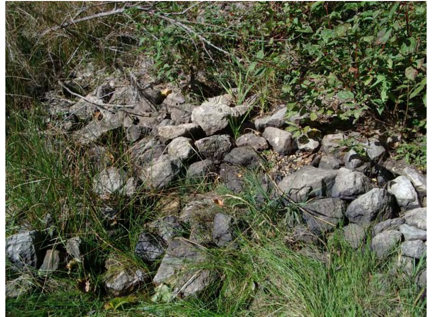
Photo 28 – View showing Wetland W7 Diffuse Discharge Inflow. Note that the gabion stone used to armour the diffuse discharge is now well-wetted, 7 years after it was installed. GEC 2017-10-01
