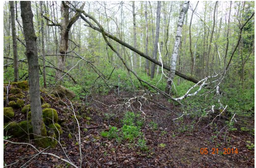
Photo 32 – View of Recharge Well RW206B, 5 years after installation in 2009. Note the woody debris and regeneration of Chokecherry, Zig-Zag Goldenrod, sedges, violets and other groundcover species. GHD 2014-05-21
