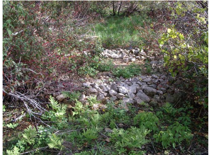
Photo 24 – View of Wetland W7 Diffuse Discharge Inflow, approximately 4 years after it was installed. Note the patch of Sensitive Fern and other wetland plants that have colonized the feeder line alignment. GEC 2014-09-22
