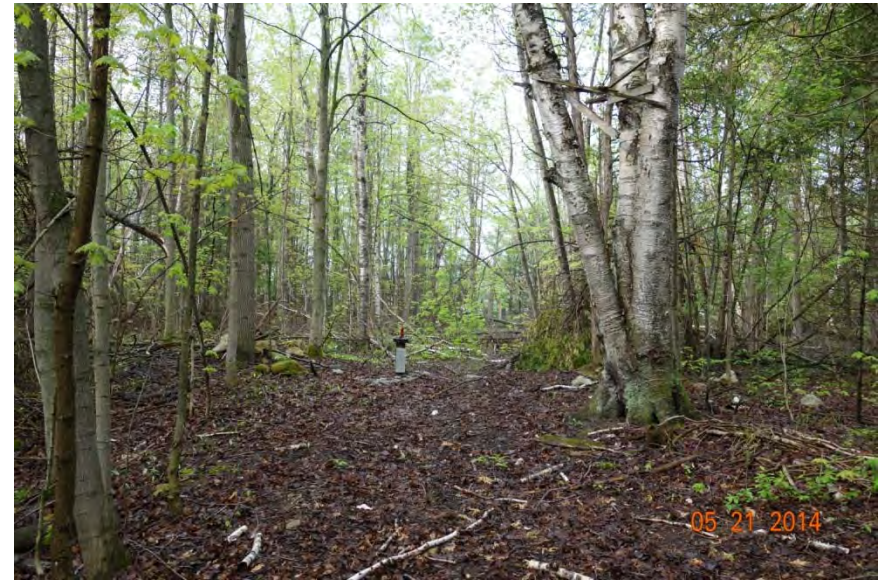
Photo 34 – View of Recharge Well RW302C, taken 3 years after installation in 2011. GHD 2014-05-21
