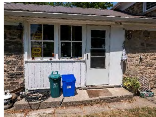
Figure 14: A former recessed porch has been enclosed on the rear wing's south face.
