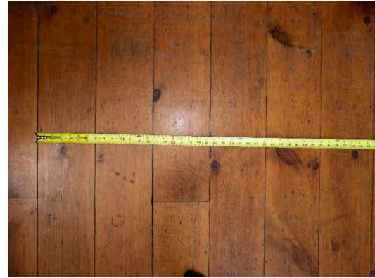
Figure 24: Pine flooring in the rear of the kitchen is of regular widths, unlike in other parts of the house.
