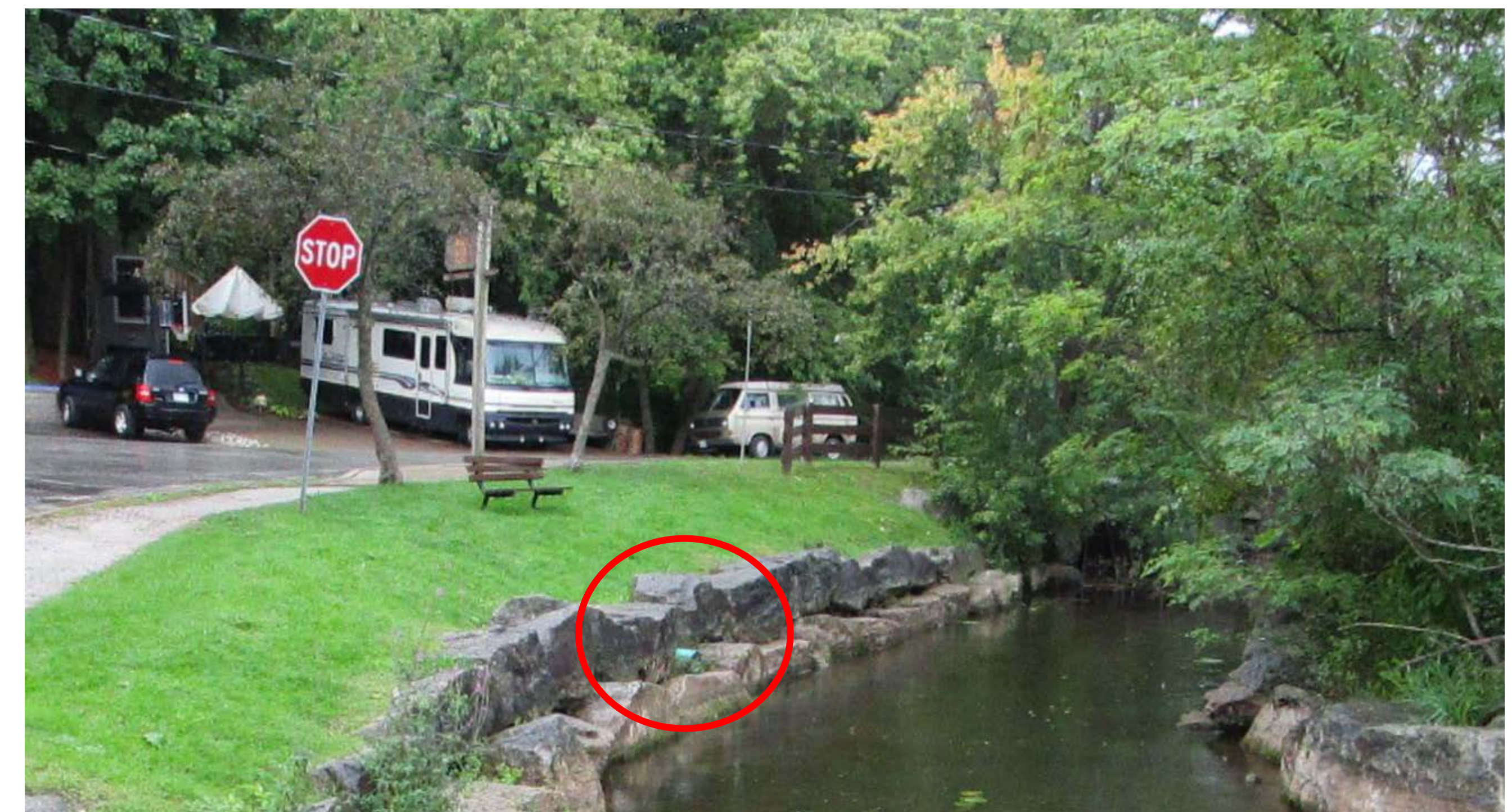
Emergency Overflow Pipe to Bronte Harbour
