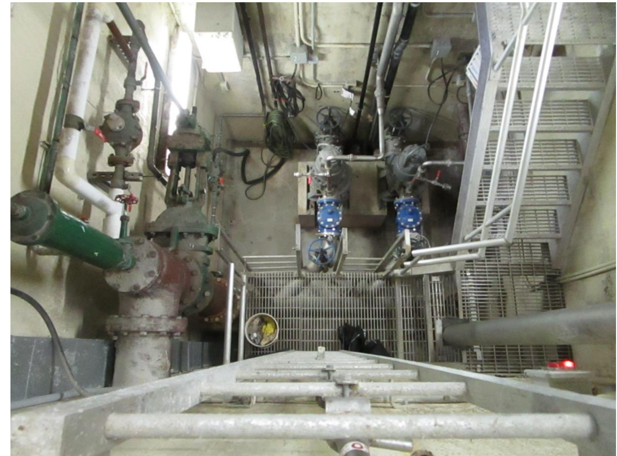
Dry Well, with view of pumps, suction and discharge piping
