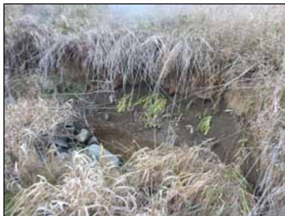
Eroding bank downstream of culvert outlet
