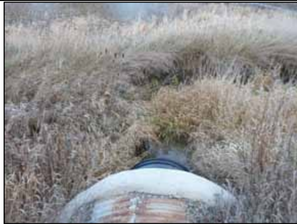
View downstream of outlet and eroding bank
