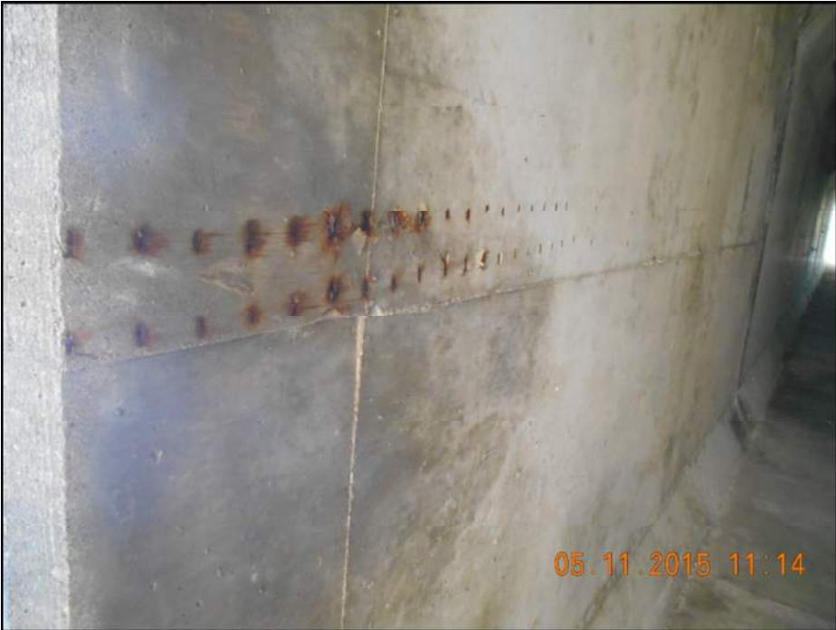
Photo 15: Rust Staining on Soffit
