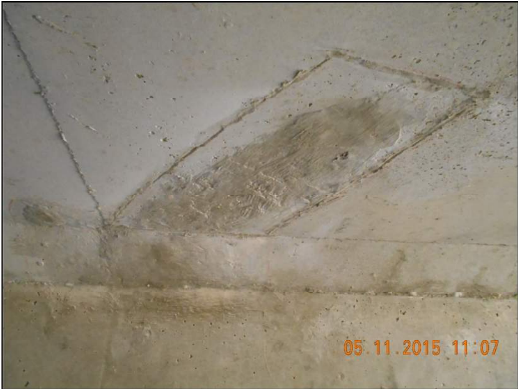
Photo 14: Saw cut in soffit not patched
