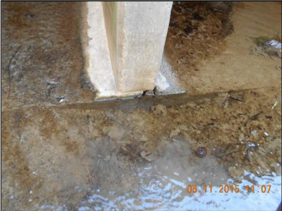
Photo 13: East end minor scour
