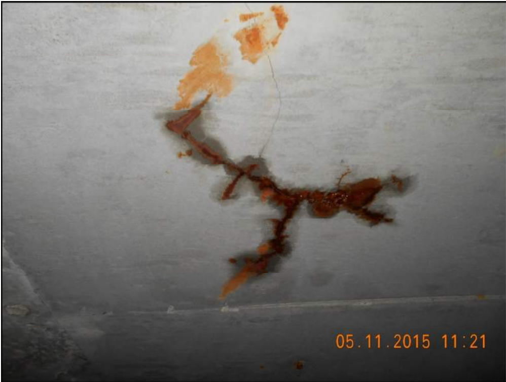
Photo 11: Crack and staining in patch repair (delaminated)
