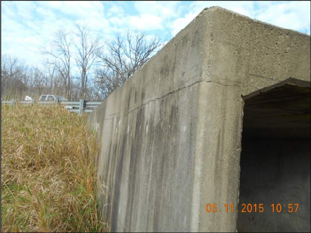
Photo 9: Full depth crack at top of wall (full exposed length)
