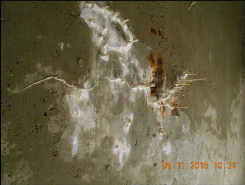
Photo 3: Efflorescence and wet staining
