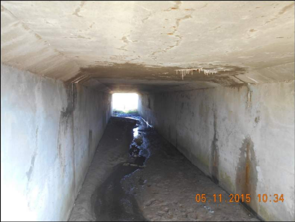
Photo 4: Wet staining along barrel
