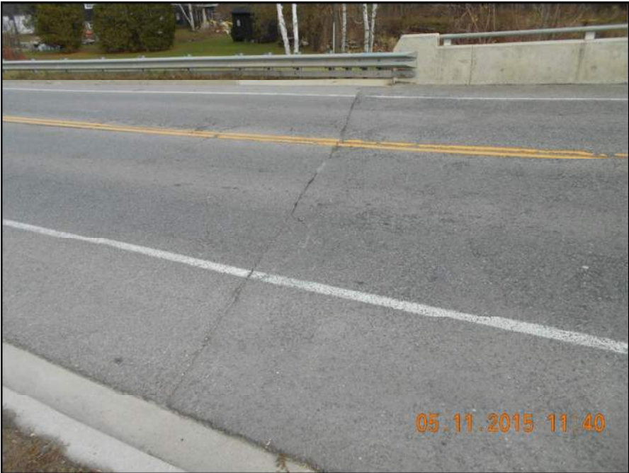
Photo 10: Unsealed Crack at North Approach (typical)
