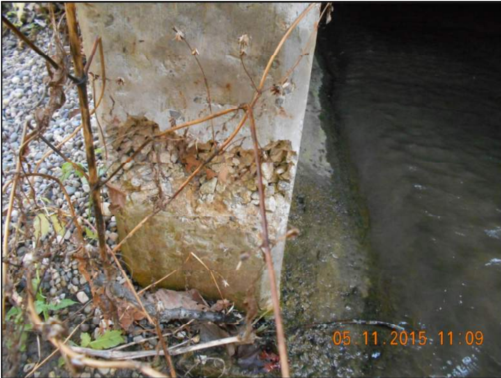
Photo 12: Spall in southeast wall face
