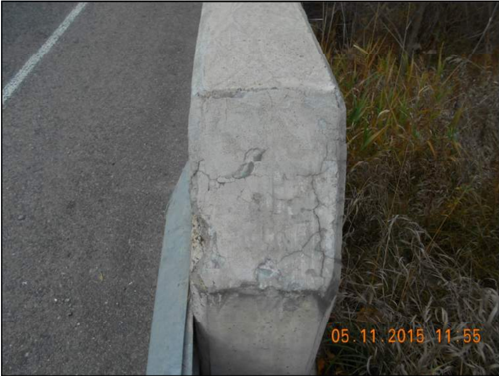
Photo 9: Southeast Delaminated Barrier
