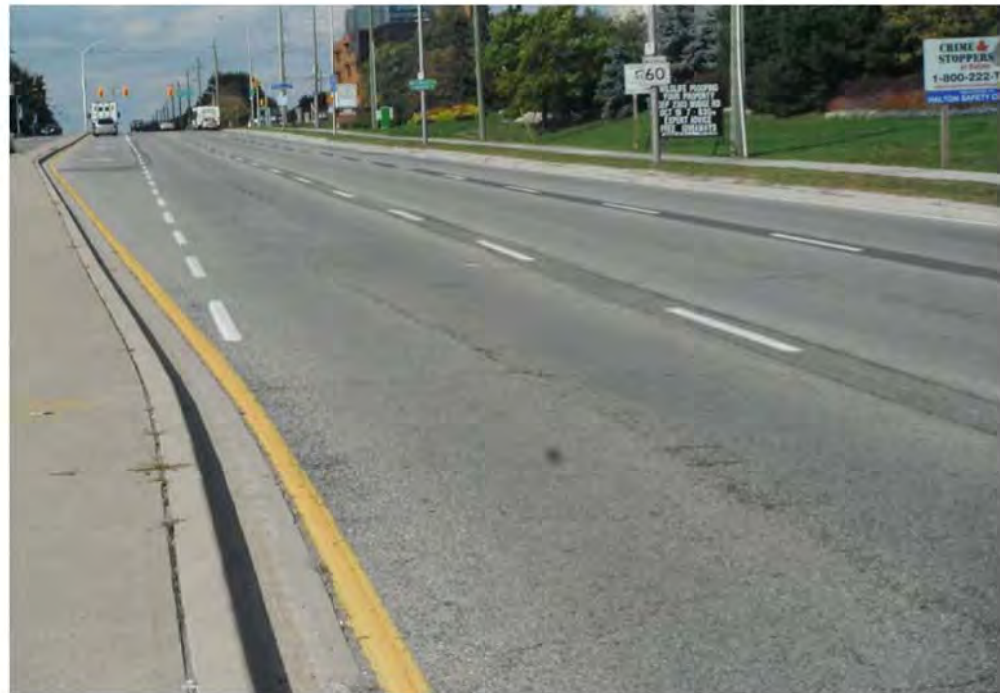
PHOTOGRAPH 1. Trafalgar Road, Section 1, showing moderate longitudinal (loading associated) and transverse cracking, slight raveling and patch repair for longitudinal construction joint cracking.
