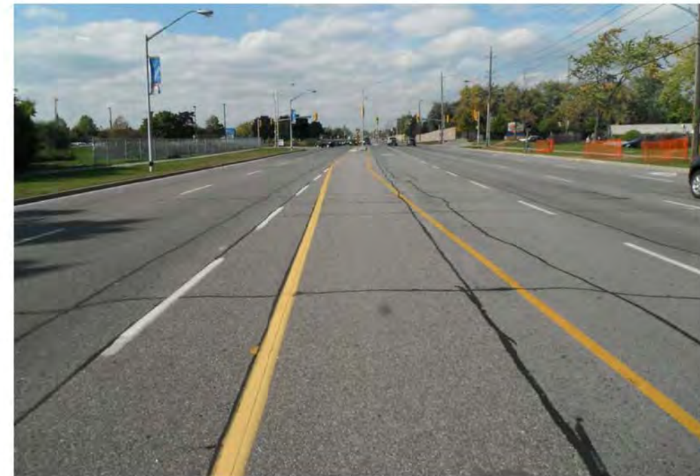
PHOTOGRAPH 4. Trafalgar Road, Section 2, showing slight longitudinal and transverse cracking sealed.
