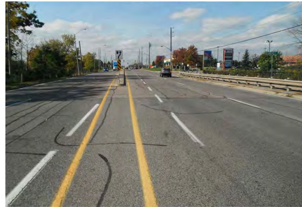
PHOTOGRAPH 7. Trafalgar Road, Section 2 approaching Dundas Street East, showing slight to moderate longitudinal and transverse cracking.
