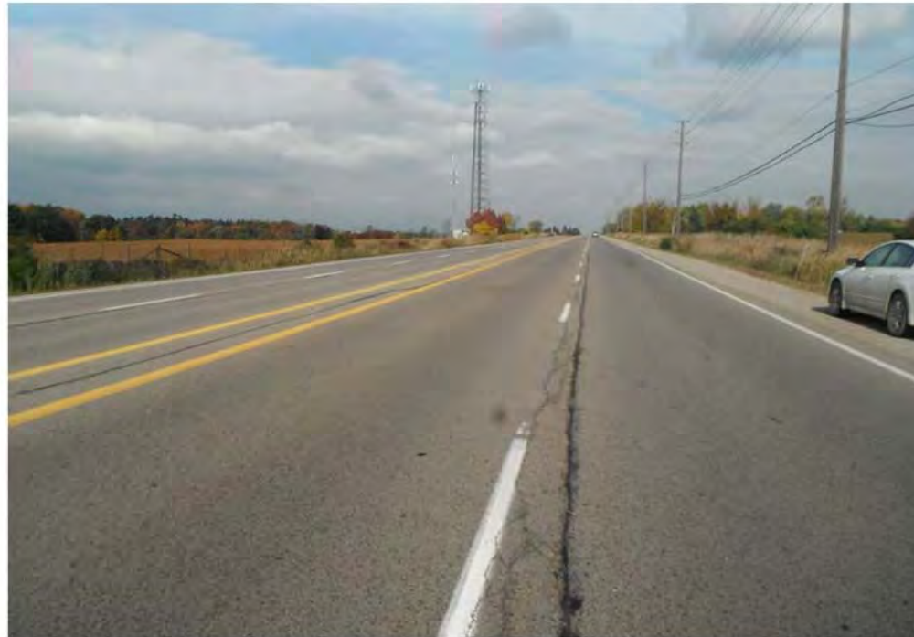
PHOTOGRAPH 9. Trafalgar Road, Section 3, showing moderate longitudinal construction joint cracking.
