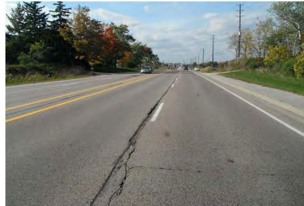
PHOTOGRAPH 11. Trafalgar Road, Section 3, showing moderate to severe longitudinal construction joint cracking.
