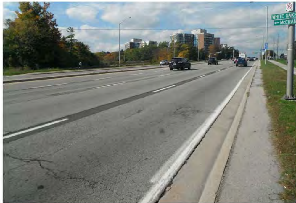
PHOTOGRAPH 2. Trafalgar Road, Section 1, showing moderate transverse cracking, slight raveling and patch repair for longitudinal construction joint cracking and drainage in fair condition.
