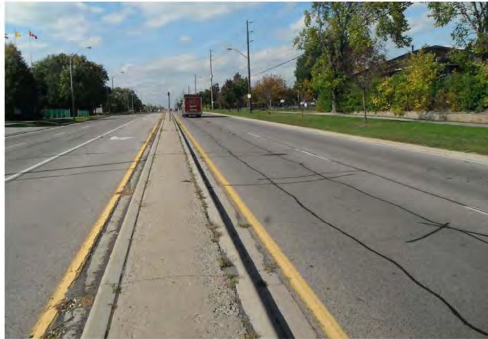
PHOTOGRAPH 5. Trafalgar Road, Section 2, showing slight longitudinal and transverse cracking sealed
