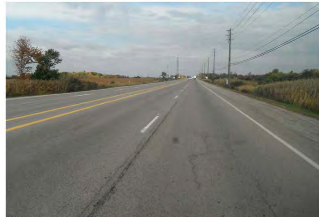
PHOTOGRAPH 8. Trafalgar Road, Section 3, showing slight to moderate longitudinal cracking
