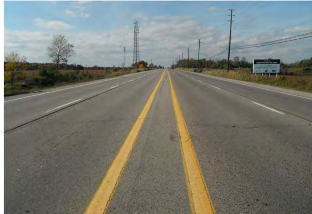
PHOTOGRAPH 10. Trafalgar Road, Section 3, showing slight to moderate longitudinal and transverse cracking.
