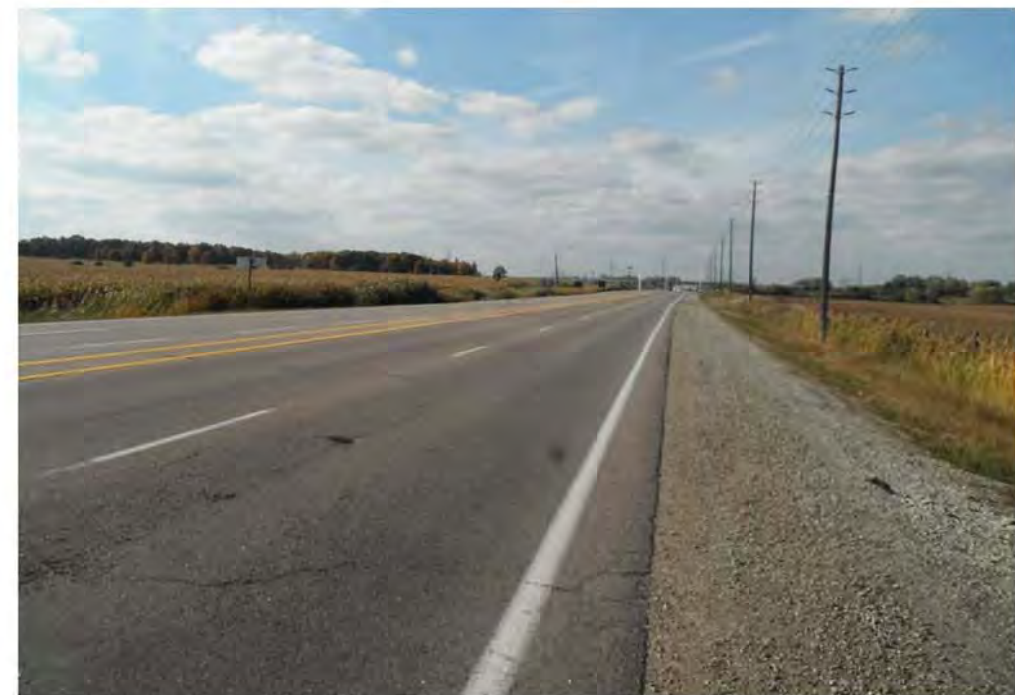
PHOTOGRAPH 12. Trafalgar Road, Section 3, showing slight transverse cracking, slight pavement edge breaks and slight lane/shoulder drop-off, side ditch with overgrown vegetation.
