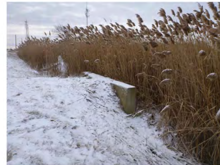
Photograph 6. East Morrison Creek – East Tributary C3 ↑ Channel is choked with vegetation on west side of culvert
