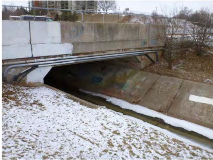
Photograph 20. Morrison Wedgewood Diversion C9 ↑ East side of concrete lined diversion channel under Trafalgar Road, captures water from several tributaries and conveys this to Sixteen Mile Creek
