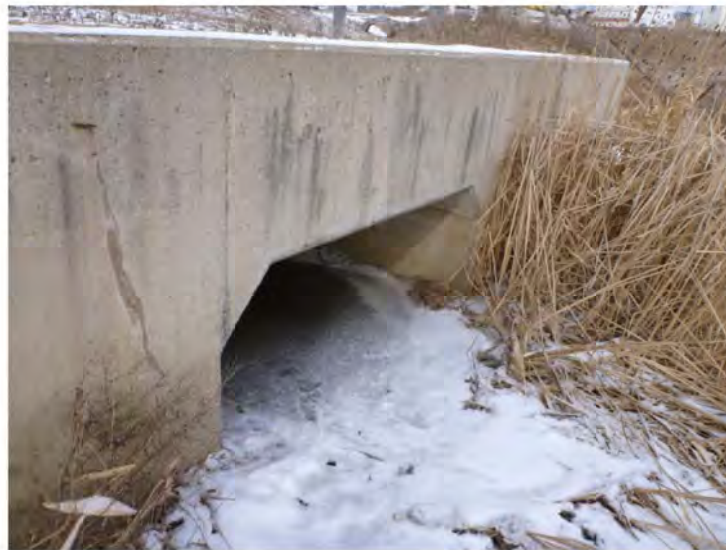
Photograph 11. East Morrison Creek – East Tributary C5 ↑ West side of culvert, conveying flow to east side
