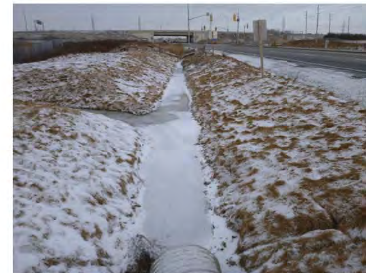
Photograph 2. Joshua Creek Crossing C1 ↑ Upstream view on west side of Trafalgar Road. Steep channel flanks GO parking lot and comes into the roadside ditch from the west side
