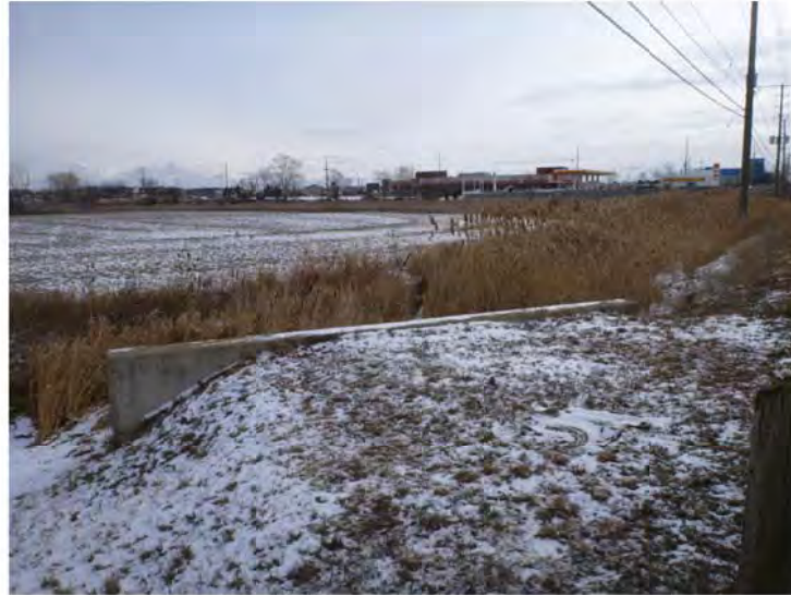
Photograph 10. East Morrison Creek – East Tributary C5 ↑ Dense vegetation occurs in channel on east side of culvert. Creek goes from west to east through culvert
