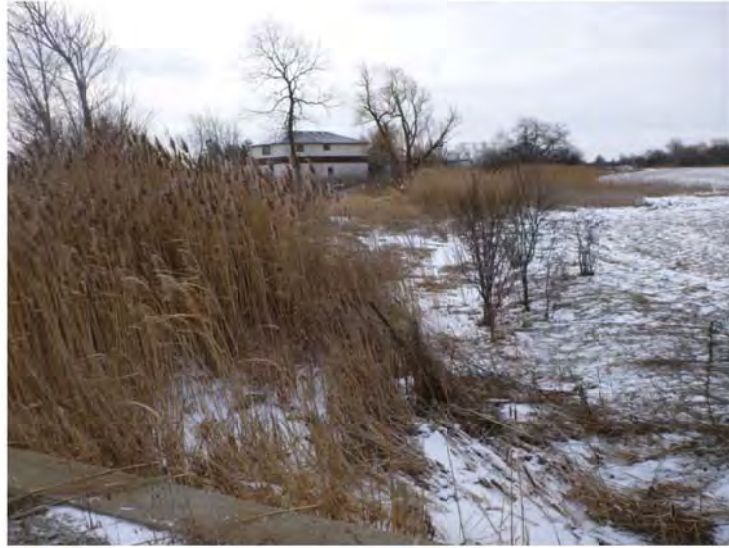
Photograph 7. East Morrison Creek – East Tributary C4 ↑ Dense vegetation occurs in channel on east side of culvert
