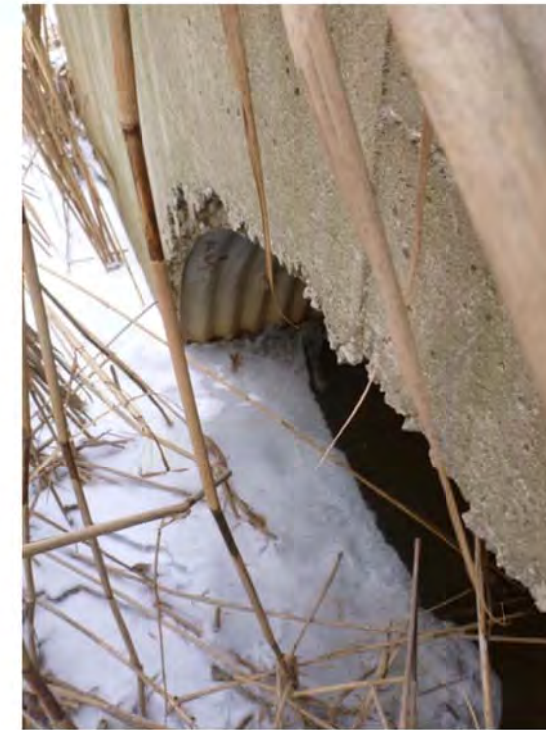
Photograph 5. East Morrison Creek – East Tributary C3 ↑ Channel is choked with vegetation on east side of culvert
