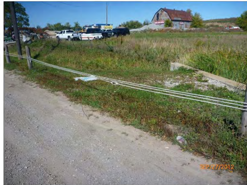
Missing Cable Guiderail Post on East Side of Structure
