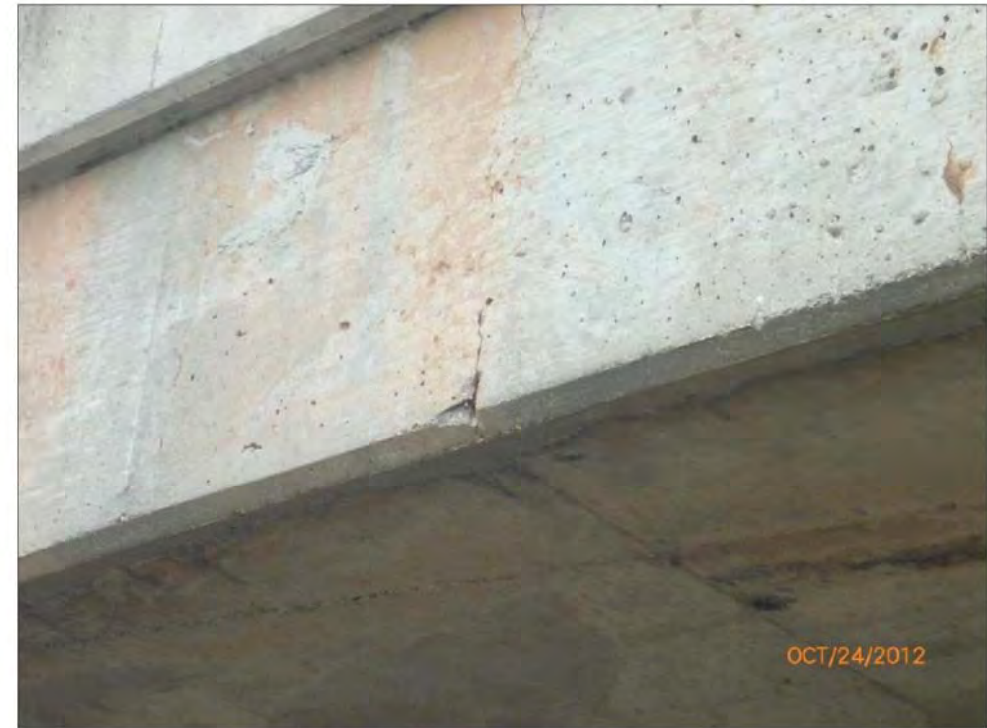
Wide Crack on Exterior Soffit
