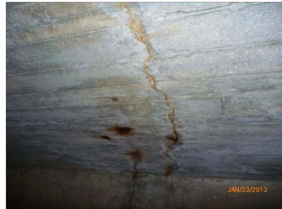
Narrow Stained Crack in Barrel Soffit
