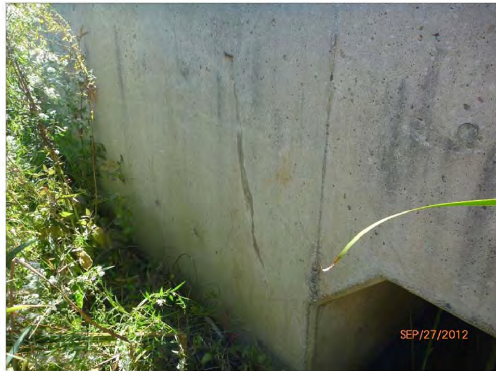
Stained Crack on Outlet Wingwall
