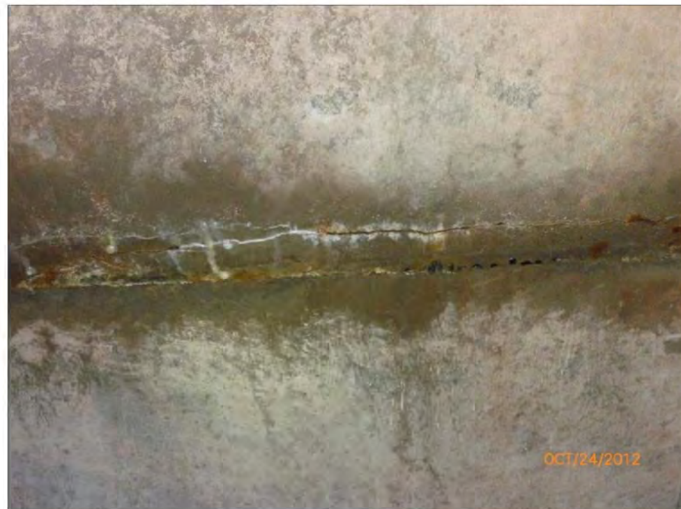
Delamination on Barrel Soffit
