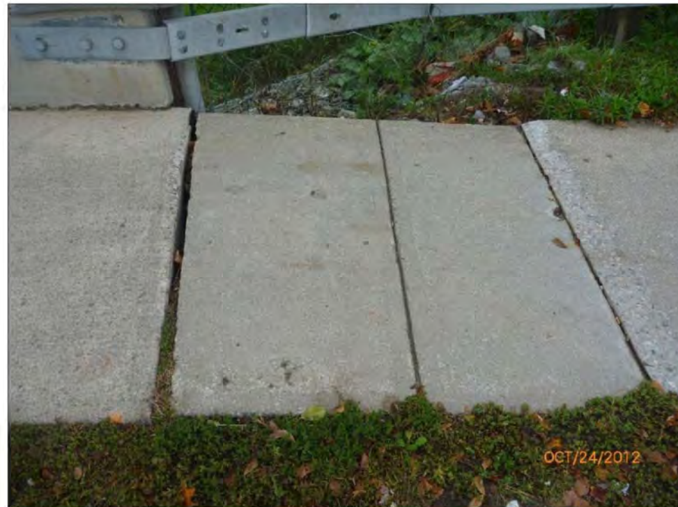
Medium Settlement of Approach Sidewalk in Southeast Quadrant
