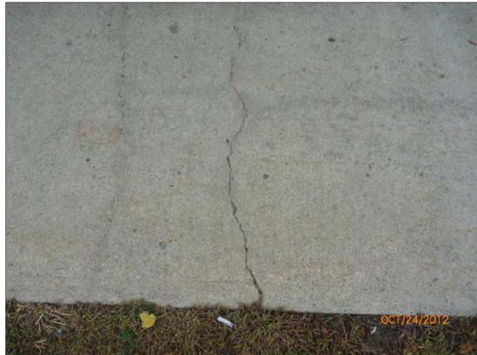
Medium Crack in Sidewalk
