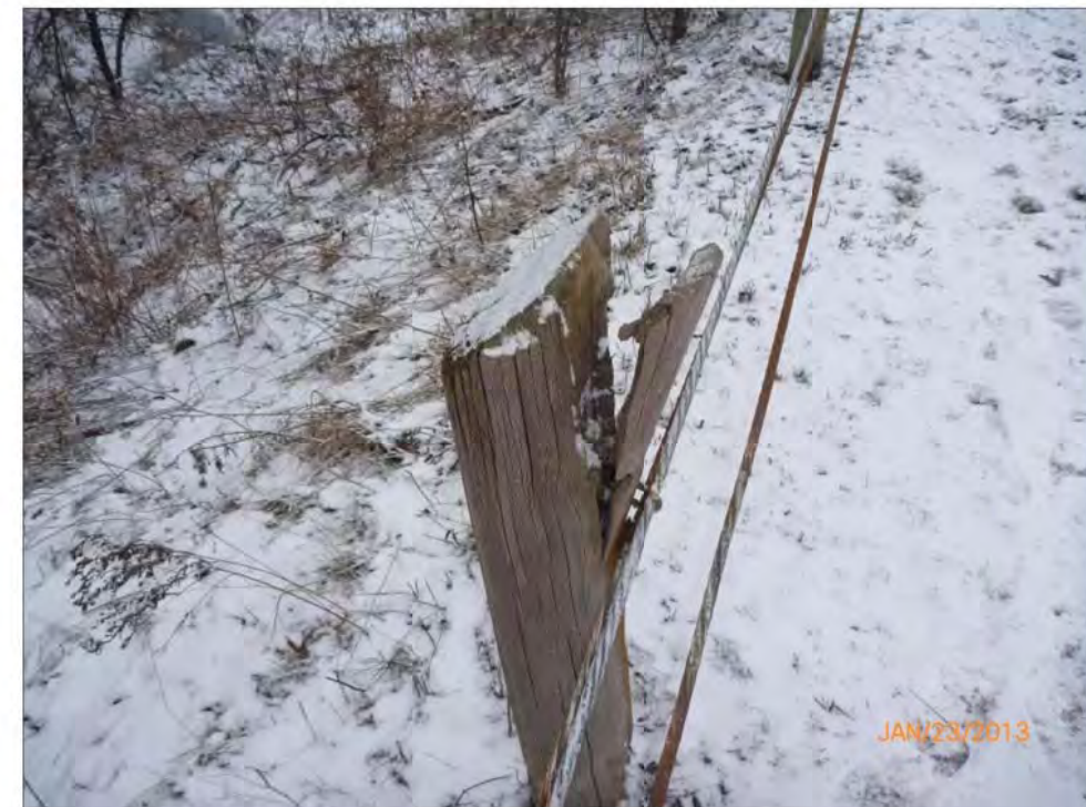
Severe Split in Timber Guiderail Post
