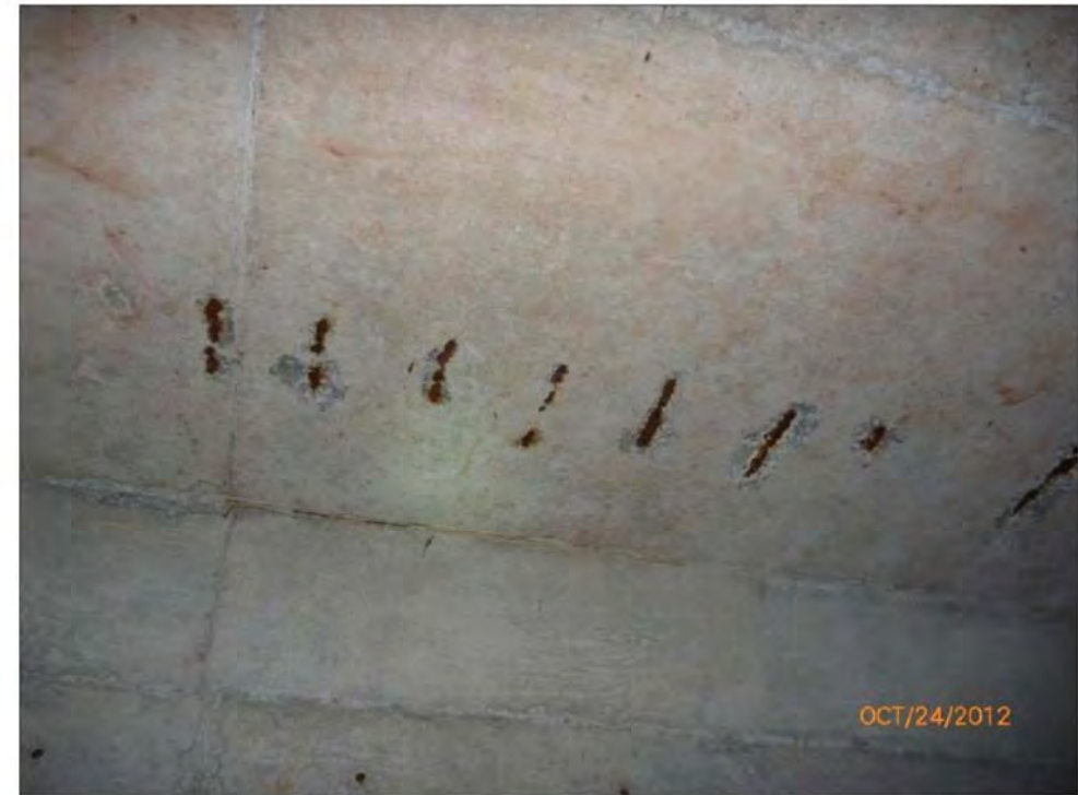
Light Spalling of Barrel Soffit
