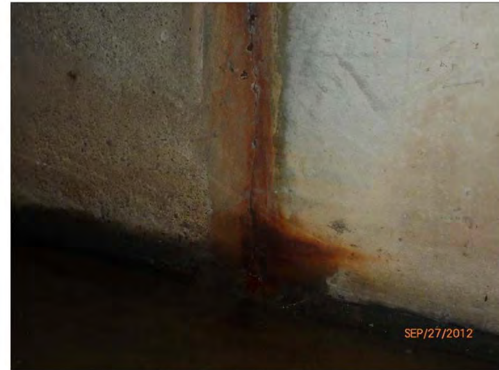
Efflorescence Staining on Barrel Wall
