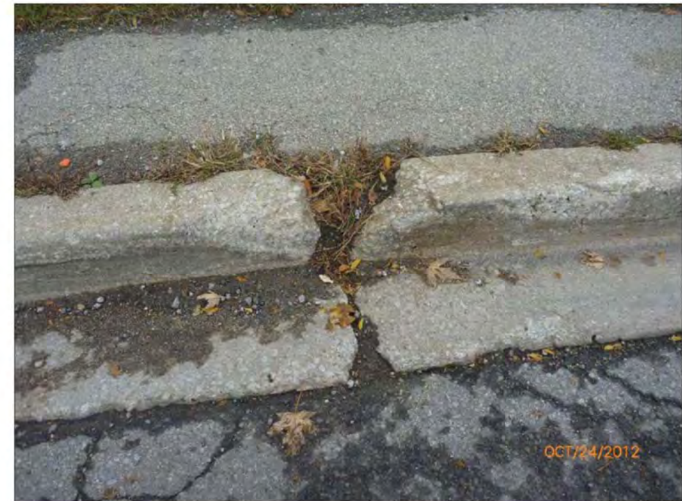
Severe Abrasion on Curb Over Deck
