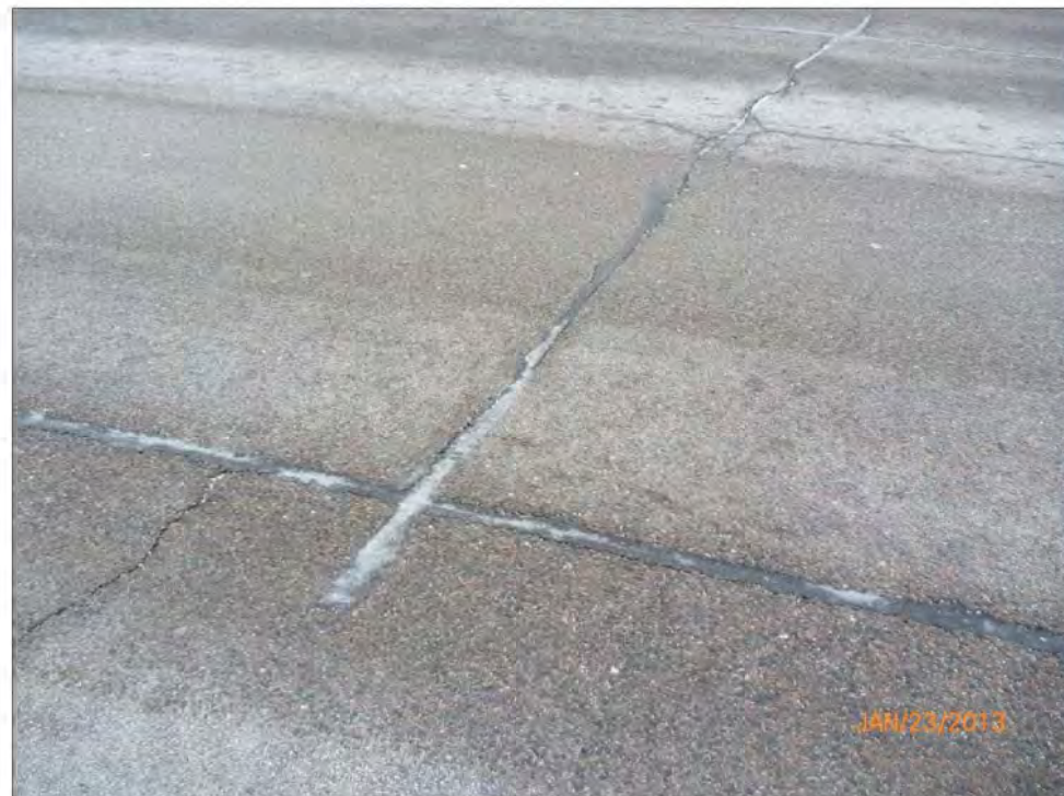
Sealed and Unsealed Narrow Cracks in Wearing Surface
