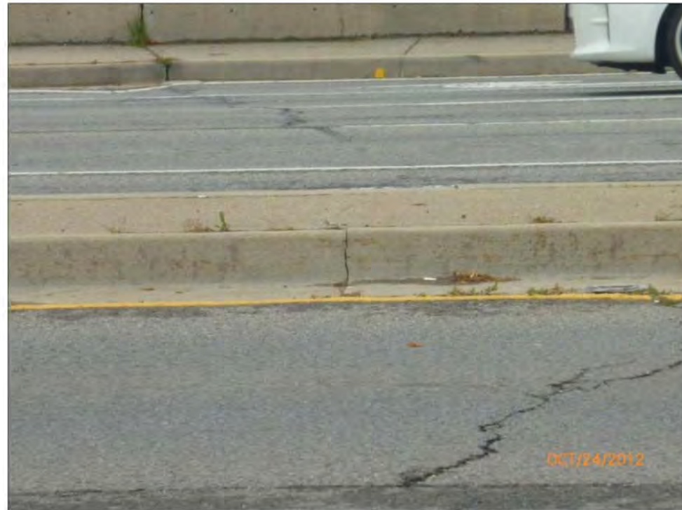
Wide Crack on Median
