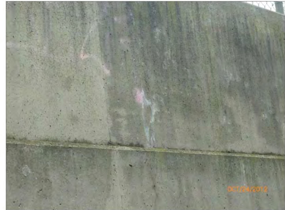
Narrow Crack on Exterior Parapet Wall
