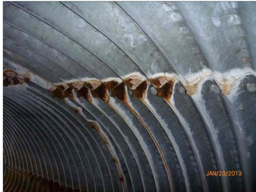
Severe Corrosion of Bolts in Barrel Obvert
