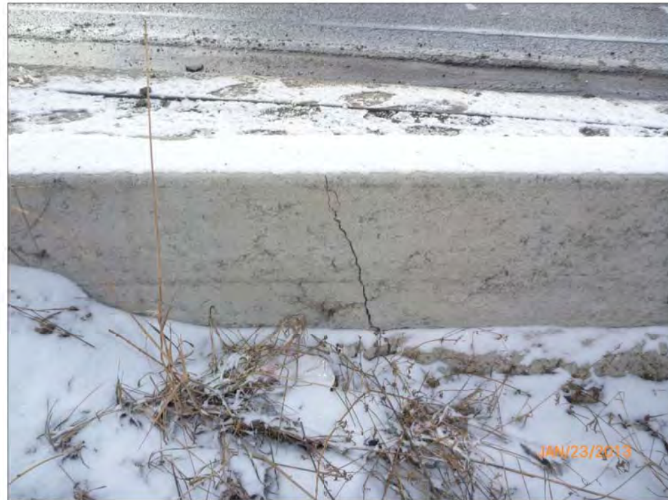
Wide Vertical Crack in East Concrete Curb
