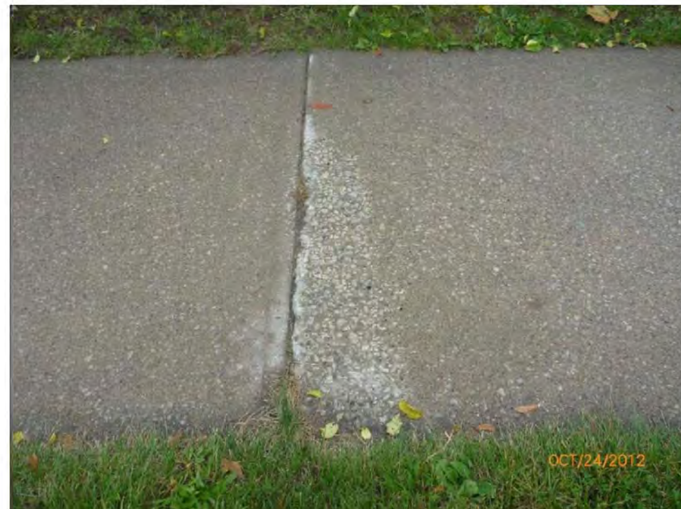
Light Scaling on Sidewalk
