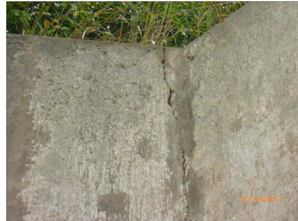
Wide Crack on Outlet Retaining Wall
