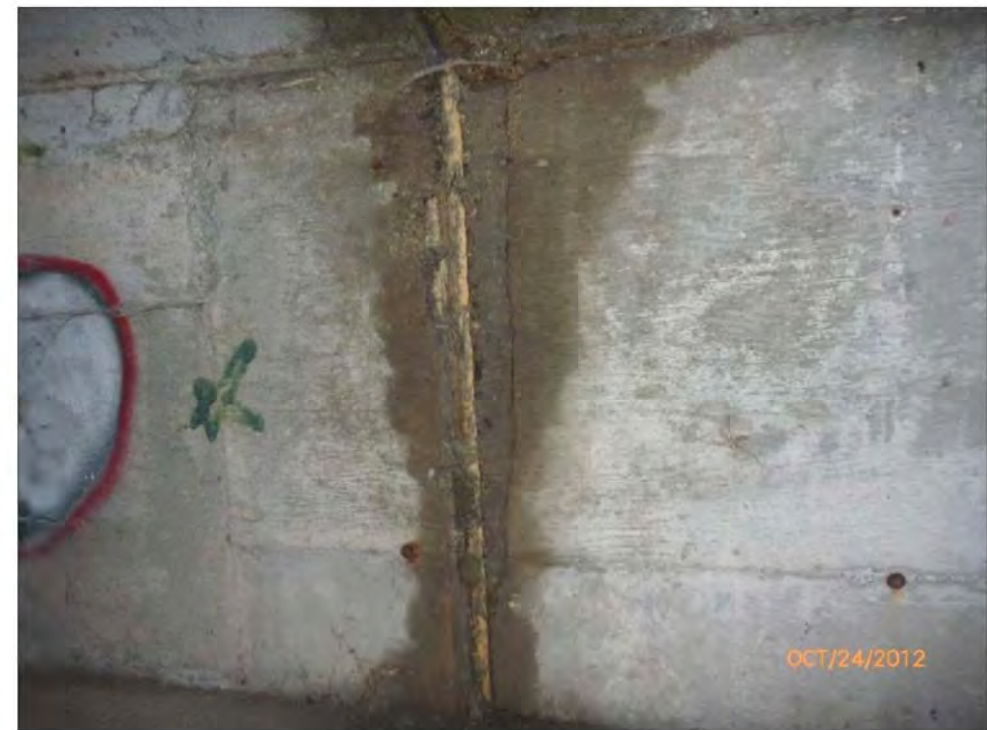
Delamination on Abutment Wall
