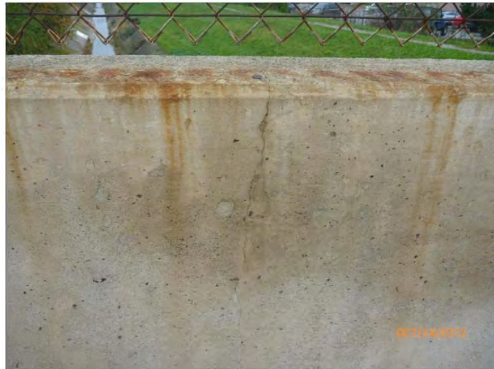
Narrow Crack on Interior Parapet Wall
