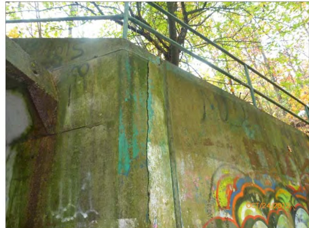
Delamination on Inlet Retaining Wall
