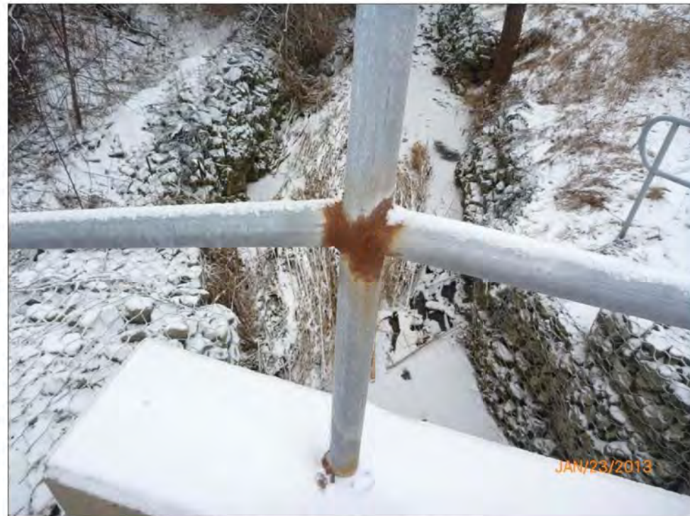
Light Corrosion of Light Pipe Handrail
