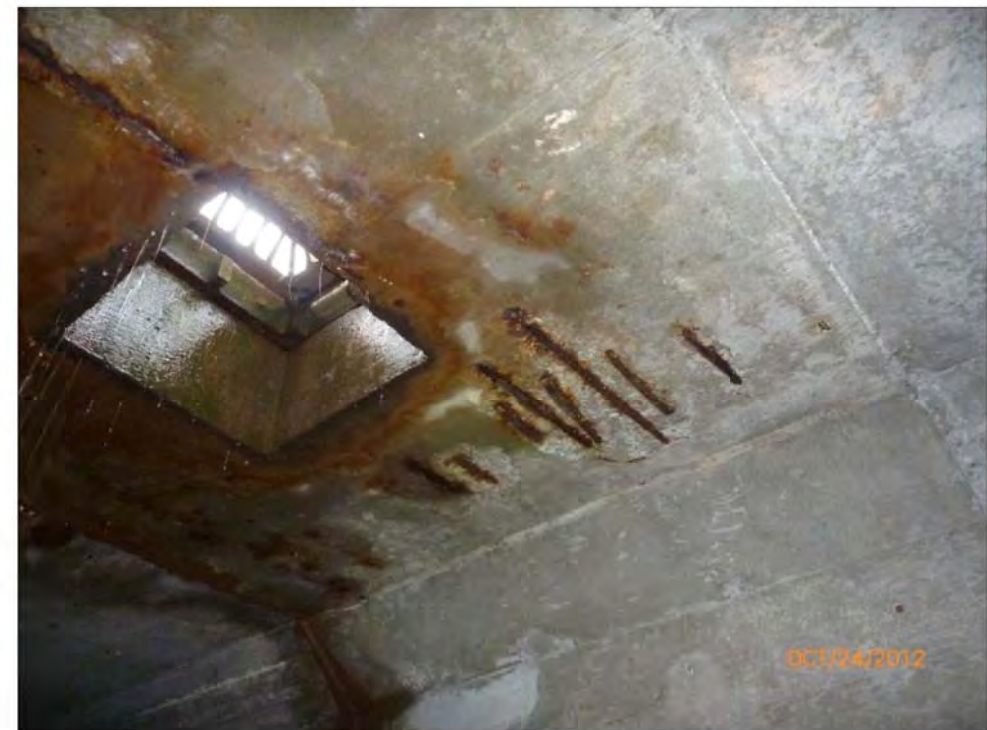
Spalling Around Storm Sewer Outlet
