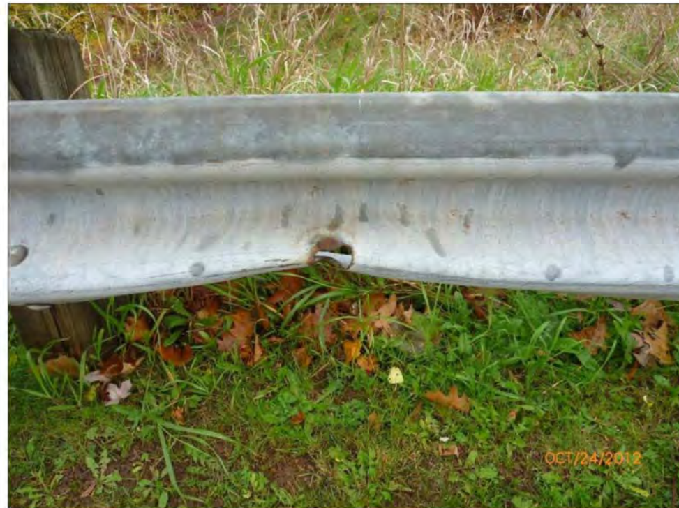
Severe Impact Damage on Flex Beam Guiderail
