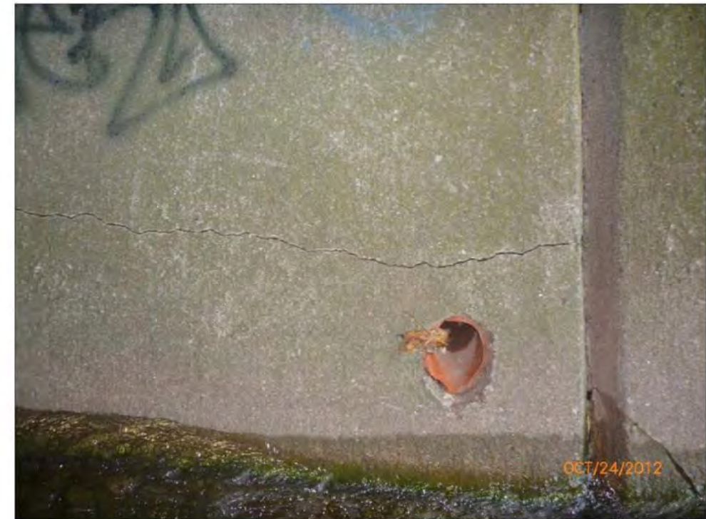
Wide Crack in Slope Protection in Front of Abutment
