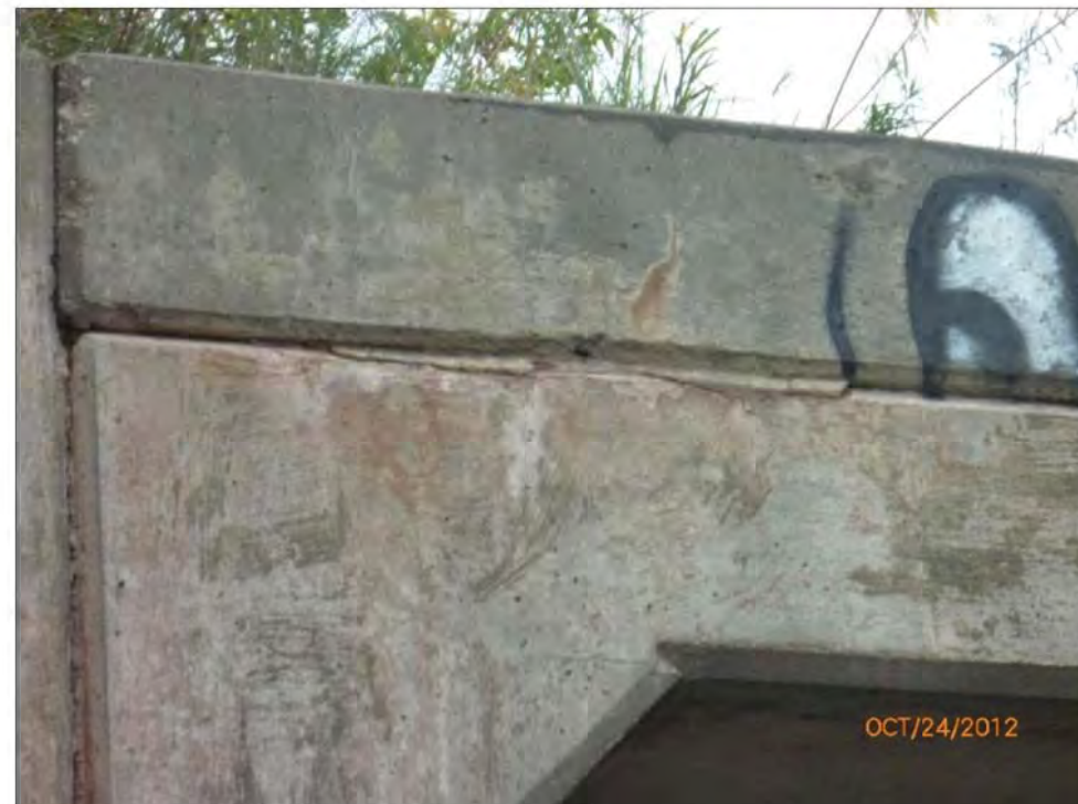
Delamination on Outlet Headwall
