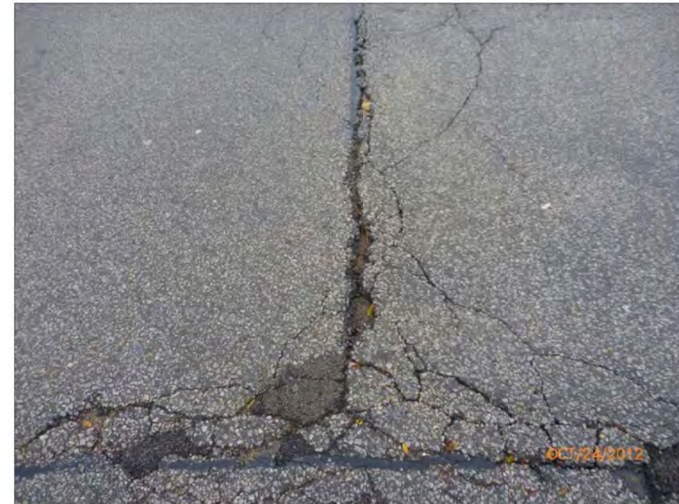
Wide Crack on Wearing Surface
