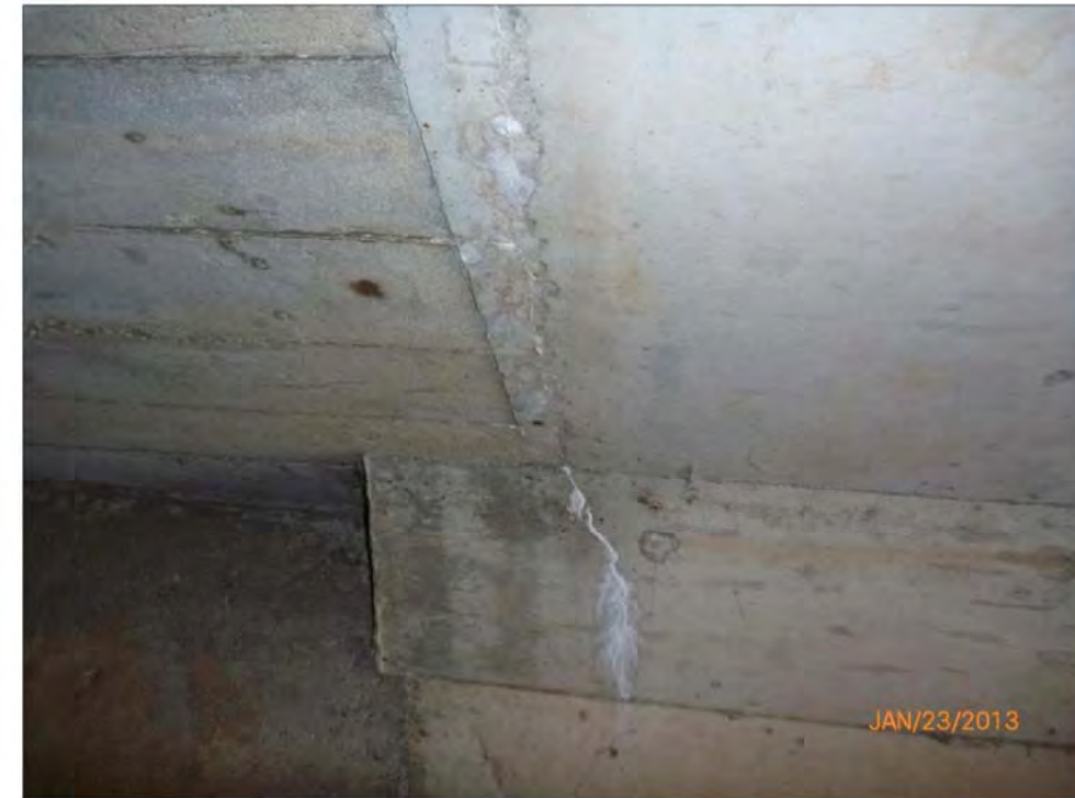
Narrow Stained Crack in Barrel Soffit Extension
