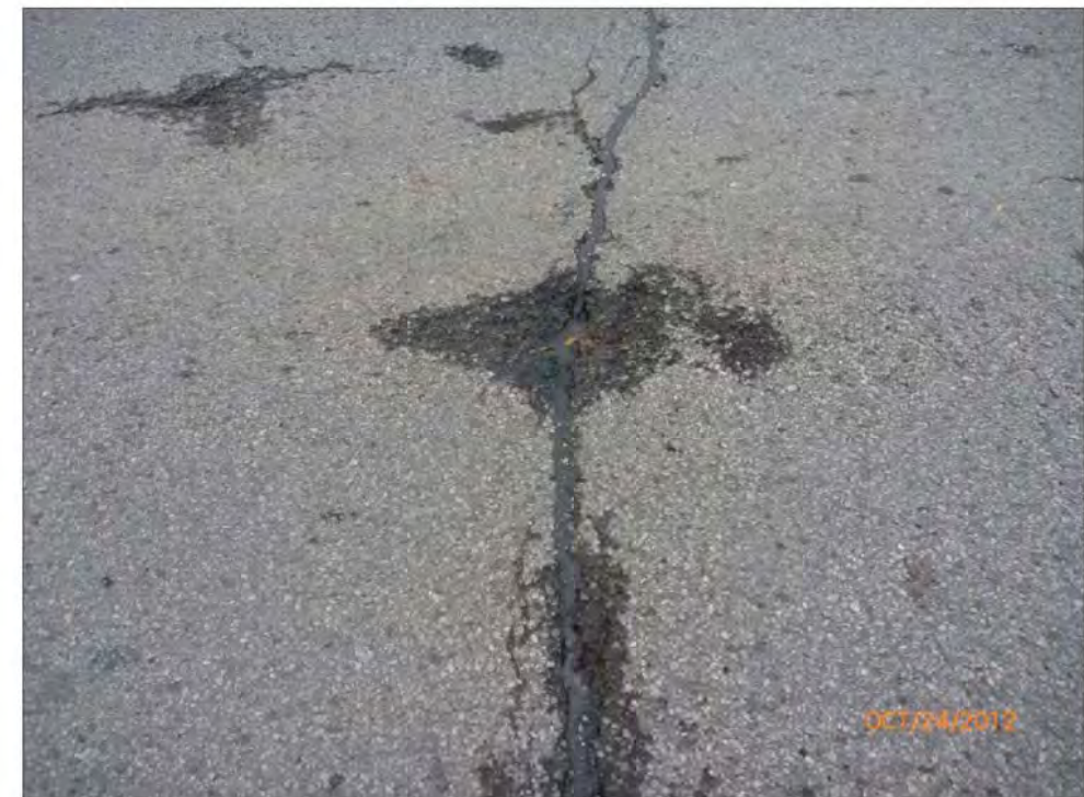
Severe Raveling of Approach Wearing Surface
