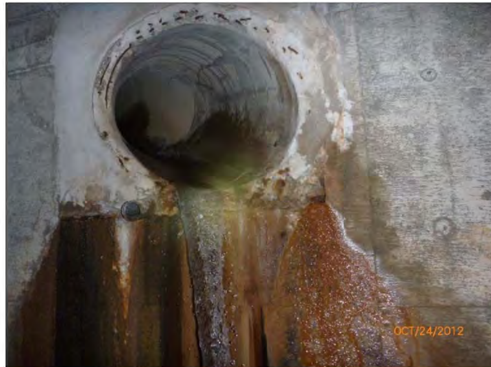
Severe Scaling Below Storm Sewer Outlet on Barrel Wall
