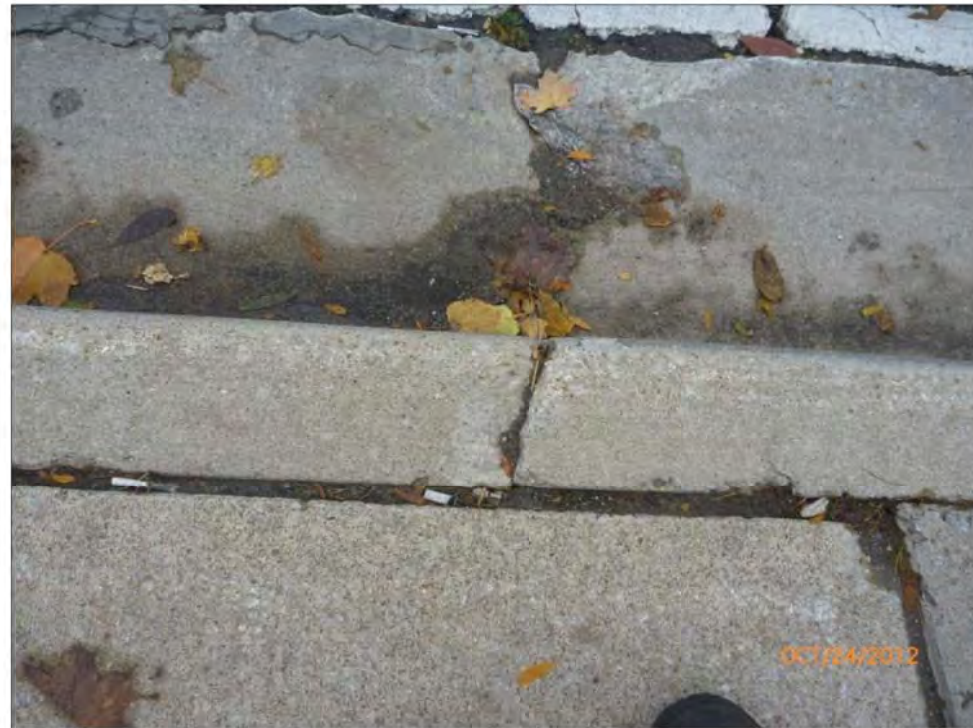
Wide Crack on Approach Curb
