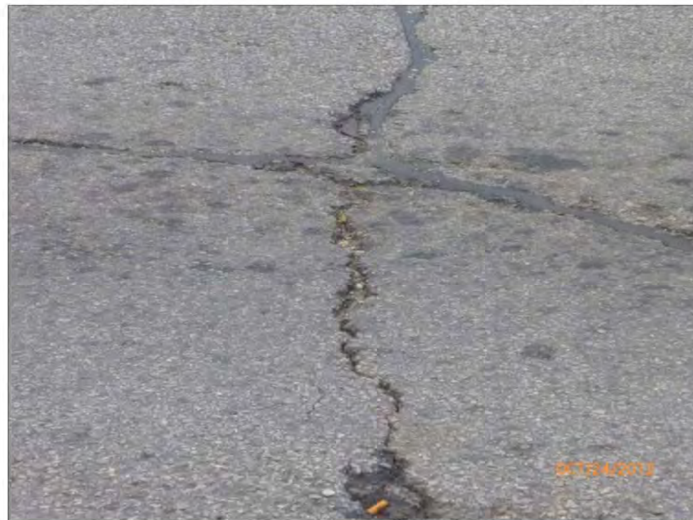
Wide Crack on Deck Wearing Surface
