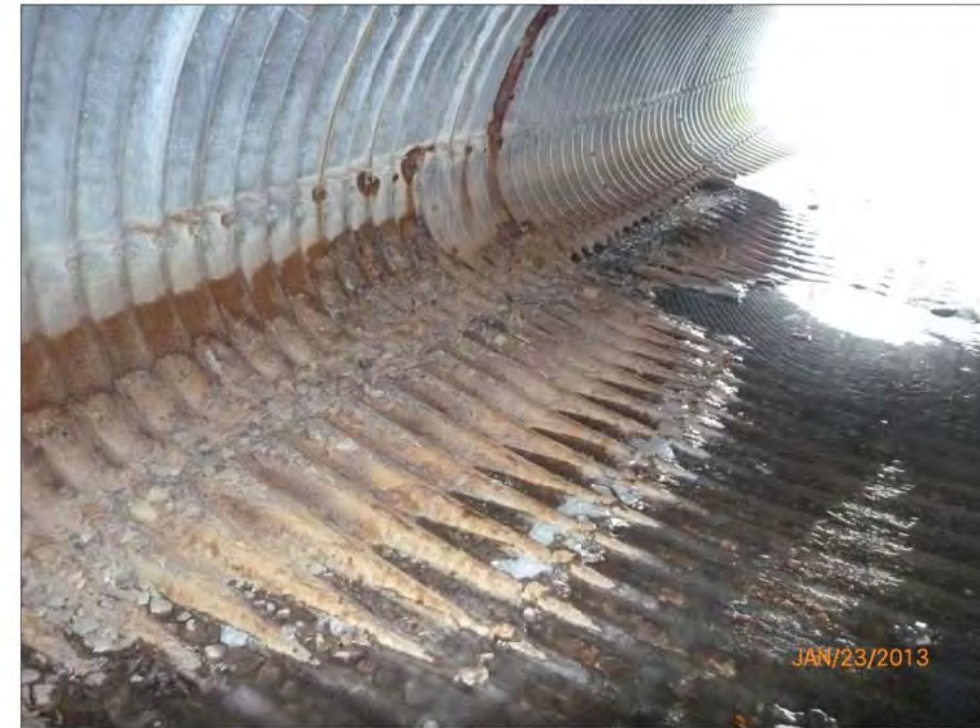
Heaving of Barrel Invert
