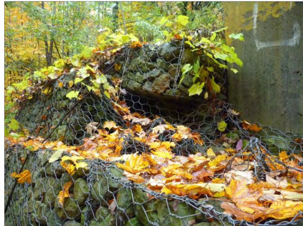
Loss of Rock at Inlet Gabion Basket
