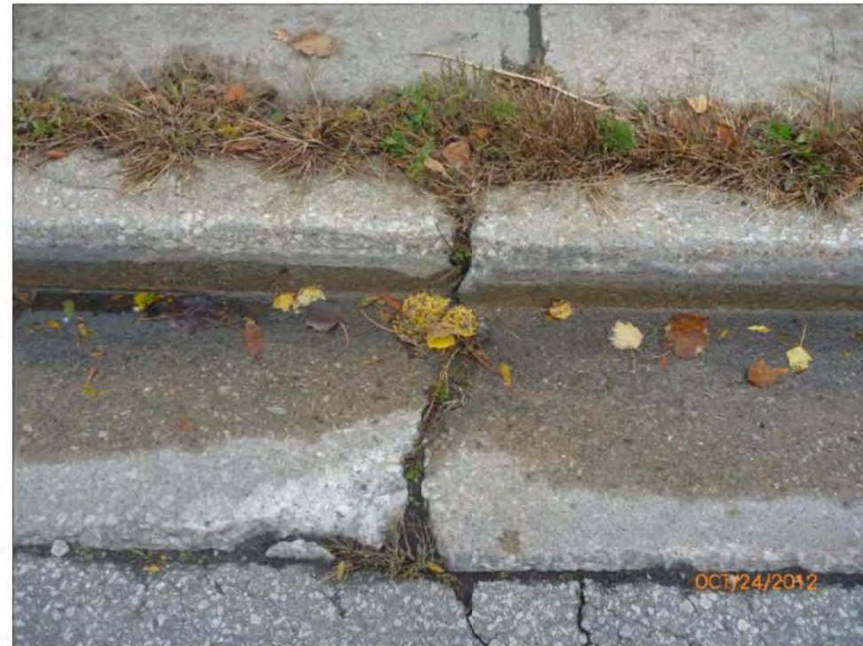
Wide Crack on Curb
