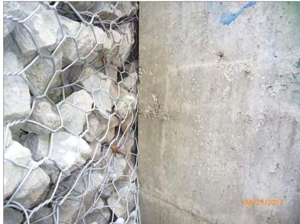
Light Honeycombing of Outlet Headwall
