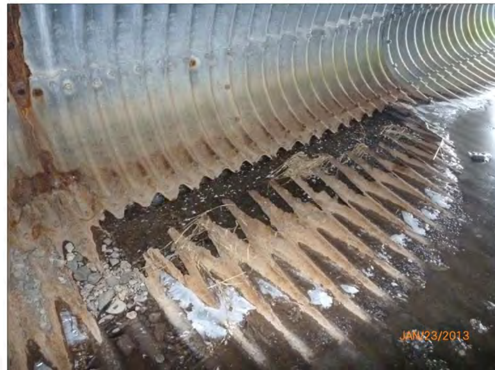
Severe Perforations in Barrel Invert
