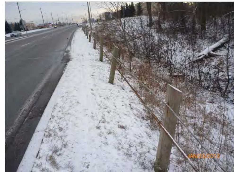
Outward Rotation of 3 Cable Guiderail (West Side)
