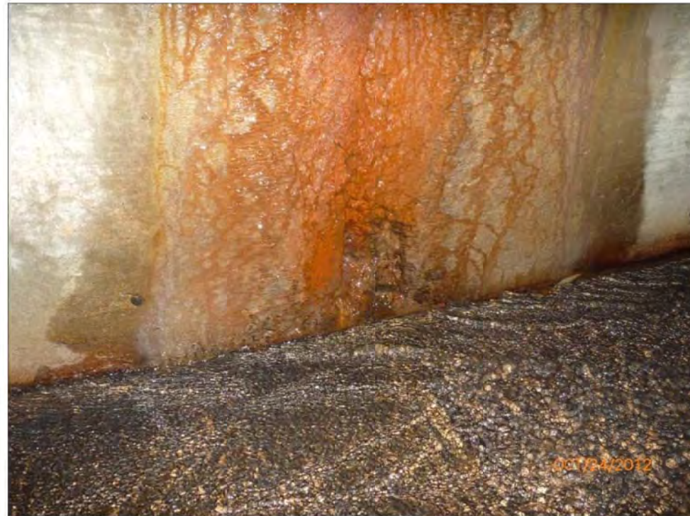
Severe Scouring of Barrel Walls
