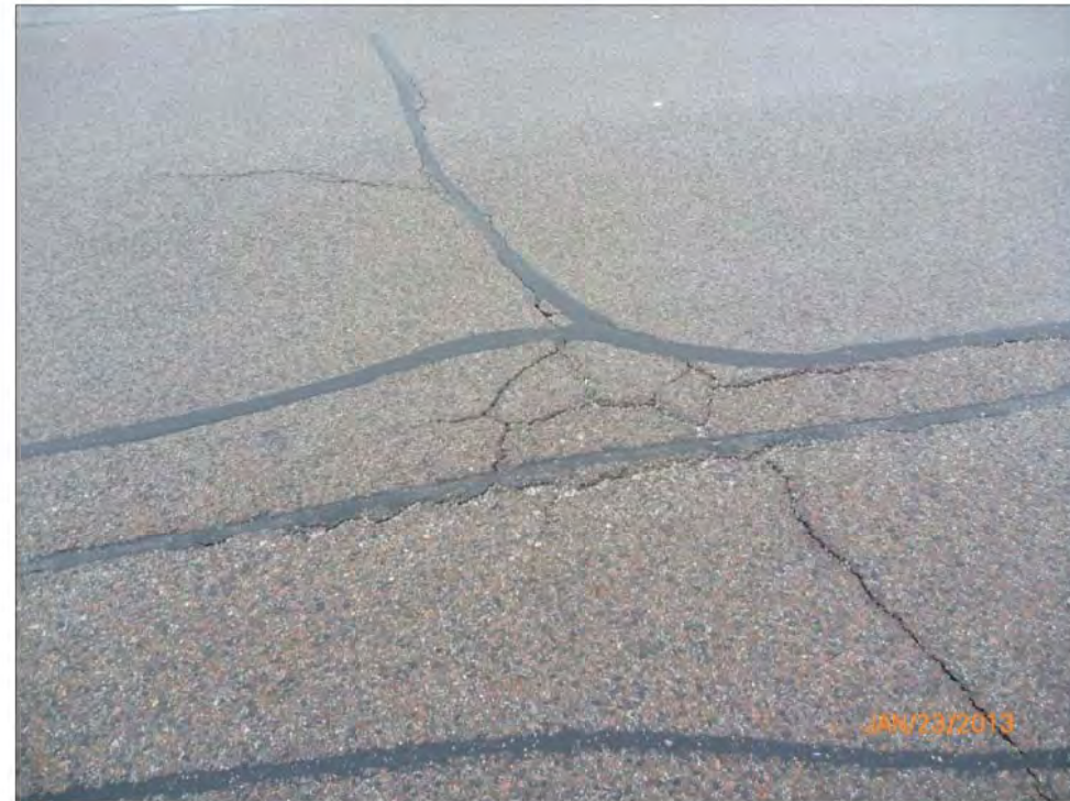
Sealed Cracks and Unsealed Narrow Cracks in Wearing Surface
