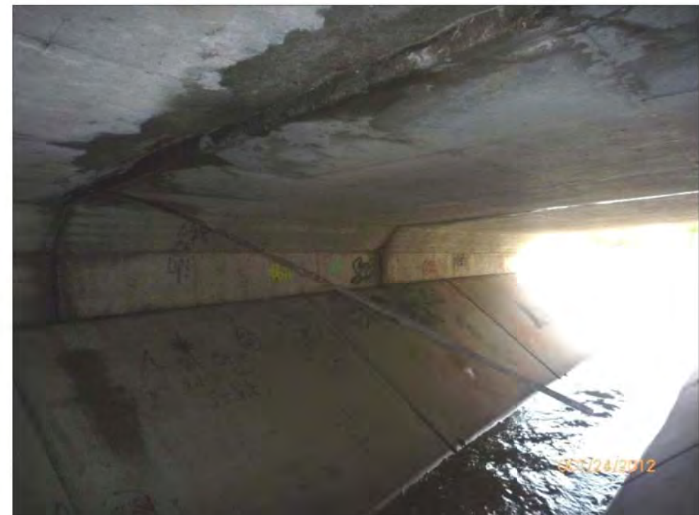
Displaced Rebar on Interior Soffit
