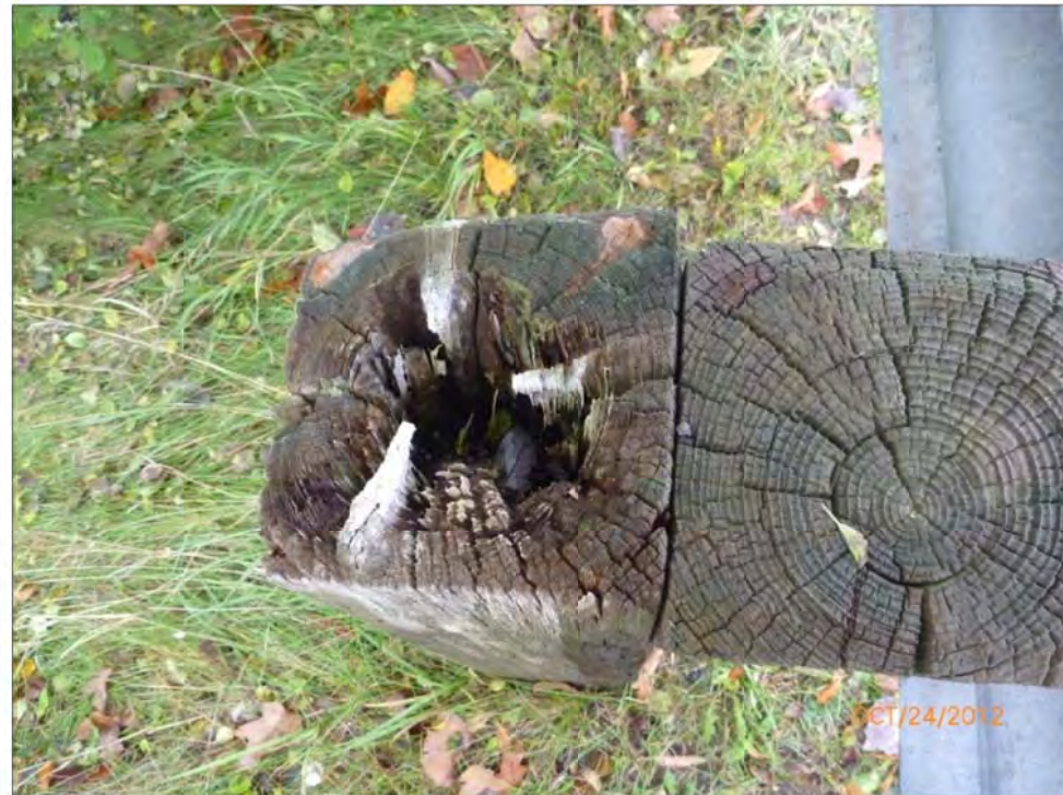
Severe End Rot on Guiderail Post
