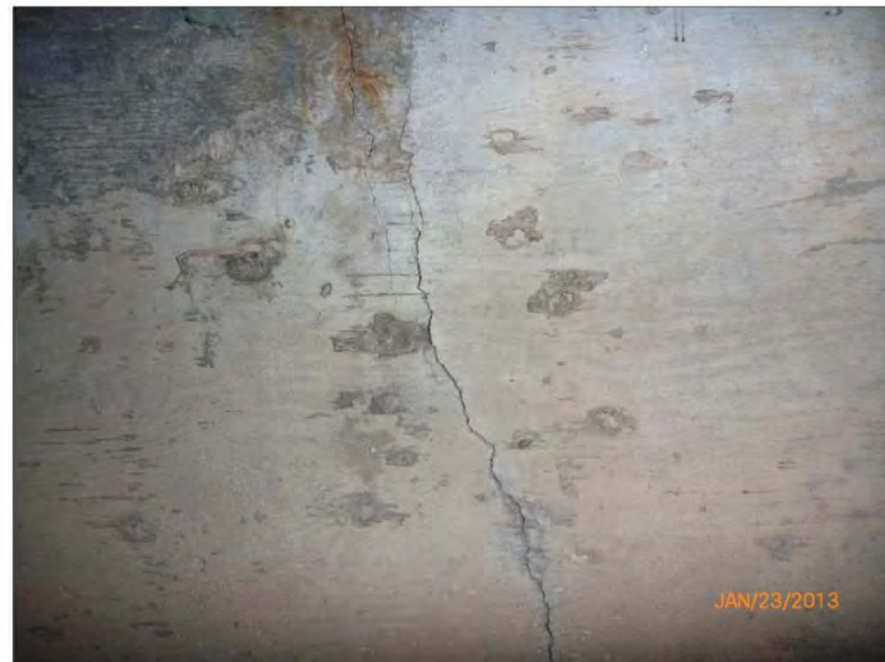
Medium Vertical Crack in Barrel Soffit
