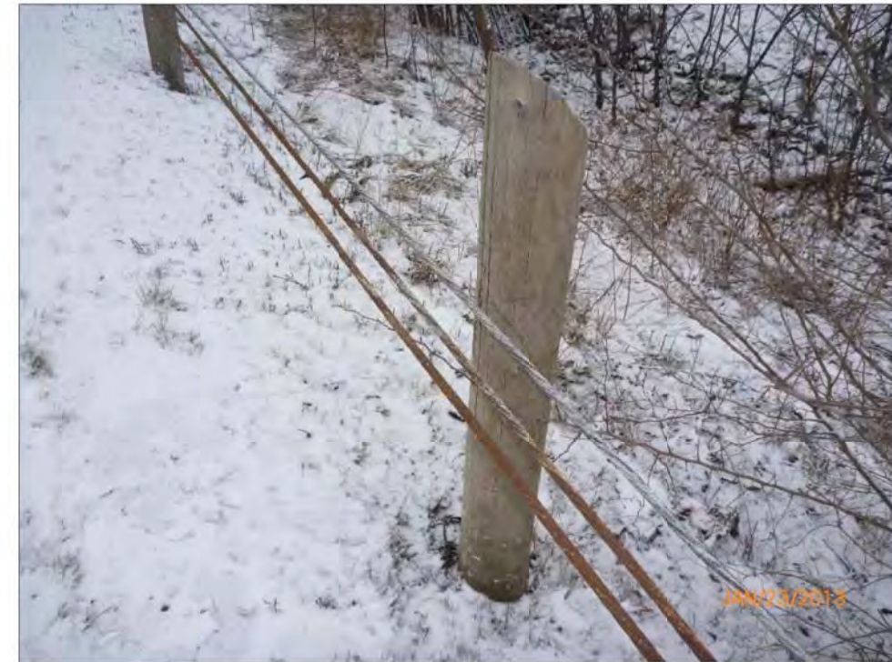
Missing Cable Stays on Timber Post
