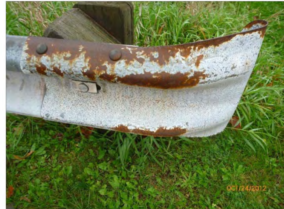
Light Corrosion on Guiderail Over Structure
