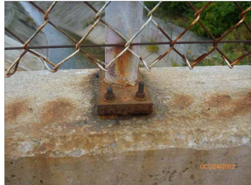
Light Corrosion on Chain Link Fence Post
