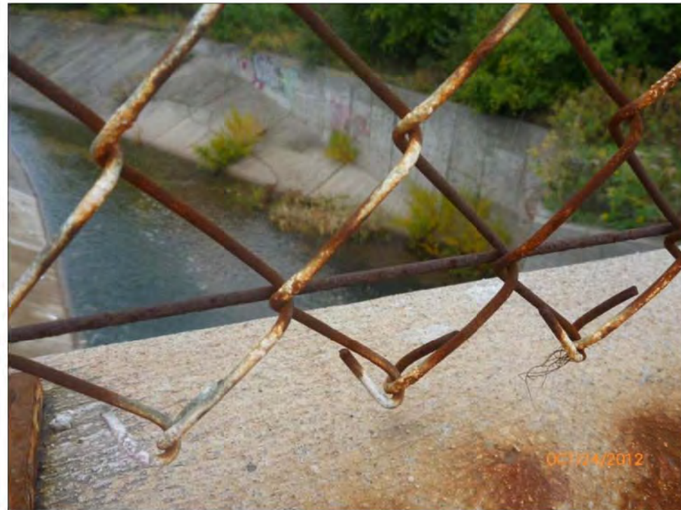
Breakdown of Galvanized Coating on Chain Link Fence
