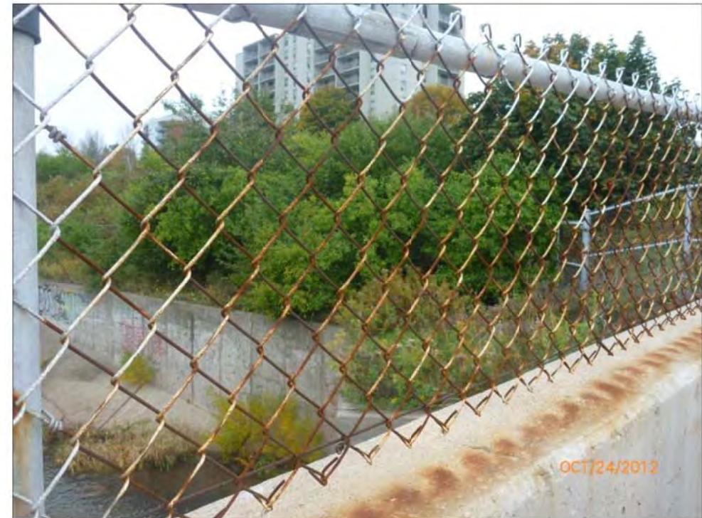
Light Corrosion on Chain Link Fence
