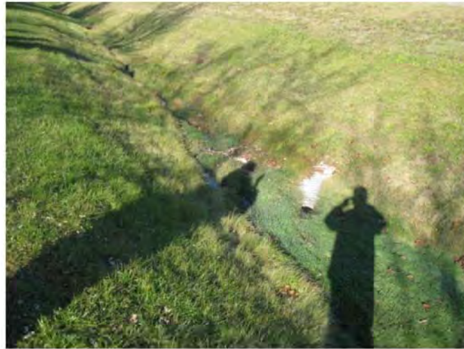
Figure 2.2 Culvert Conveying Runoff from East Roadside Ditch to West Roadside Ditch, Across Trafalgar Road
