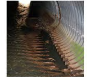
Figure 2.14 Corrosion at Culvert 5+225
