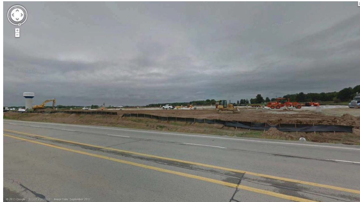
Image 12: Looking slightly southwest along Trafalgar at grading disturbance associated with development.
