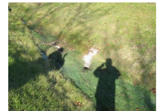
Exhibit 3-7. Culvert Conveying Runoff from East Roadside Ditch to West Roadside Ditch, Across Trafalgar Road
