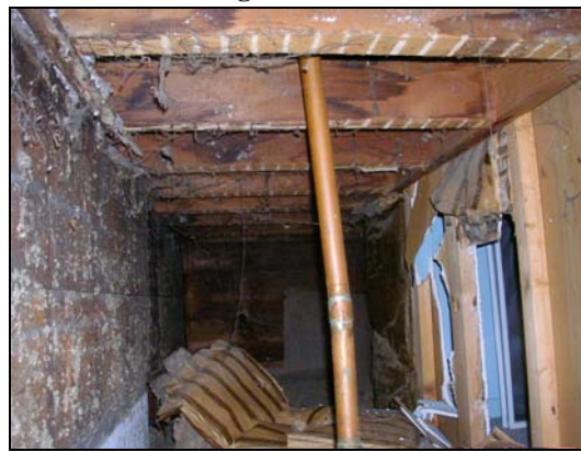
Space between knee wall and exterior south wall showing construction of new knee wall.
