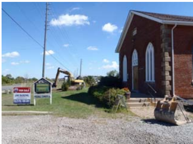
Plate 9: View northwest of study area, with St Paul's church in the foreground.
