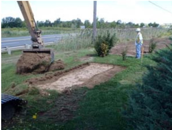
Plate 7: Monitoring of trench excavation following excavation of test pits, looking north. Note evidence of disturbance due to utility installation.
