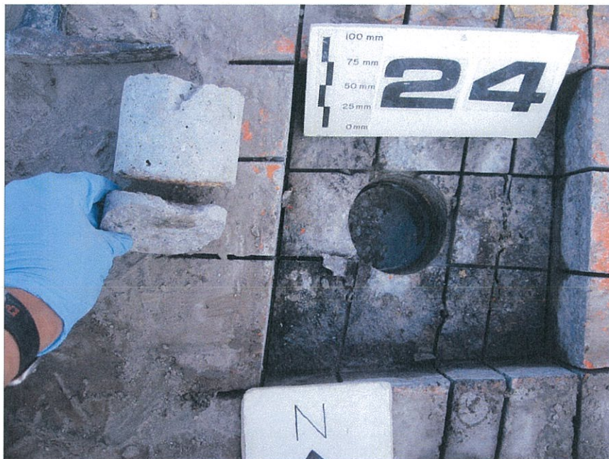
Photograph 12 – Horizontal void found within the concrete deck at sawn asphalt sample S4 (Core C24 taken at this location); construction joint between gutter and deck
