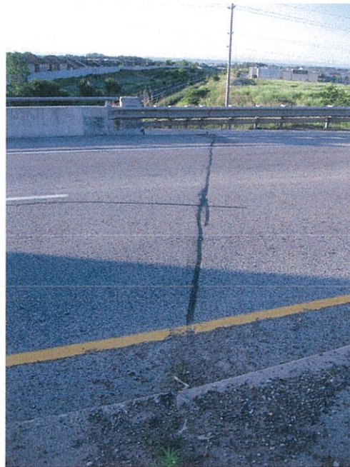
Photograph 10 – Transverse sealed crack at west approach (typical)
