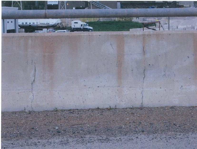
Photograph 20 – Vertical medium cracking in concrete parapet walls (typical)
