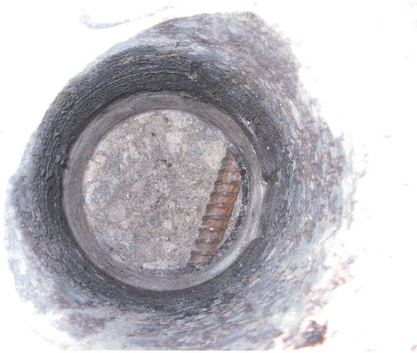
Photograph 17 – Light rust noted on reinforcing steel at eight (8) core sample locations (Core C15 shown)
