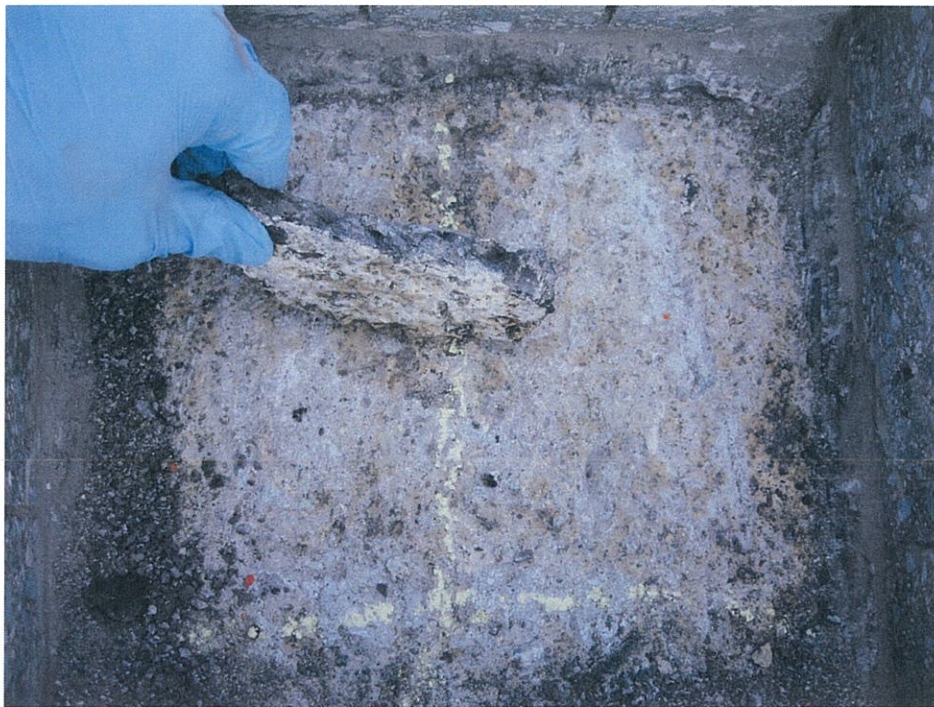
Photograph 14 – Scaling noted on concrete surface at sawn asphalt sample S5
