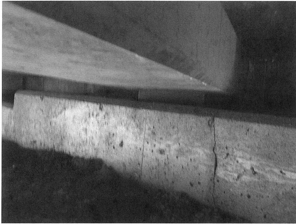
Photo 4 – Crack at West Abutment
