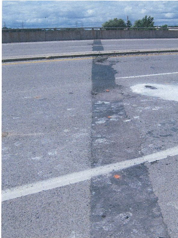
Photograph 11 – Asphaltic plug seal applied over east pier expansion joint, looking north (typical); Note the patched areas and voids in the plug seal
