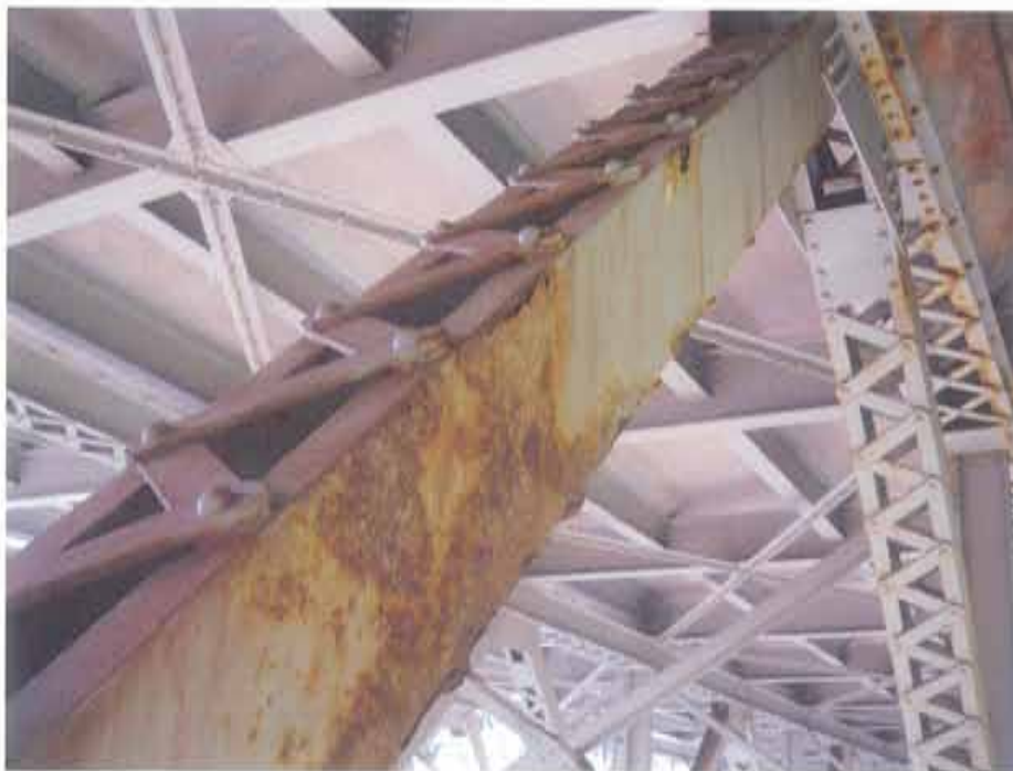
Photograph 62. Typical medium corrosion noted in diagonal and vertical members of T1
