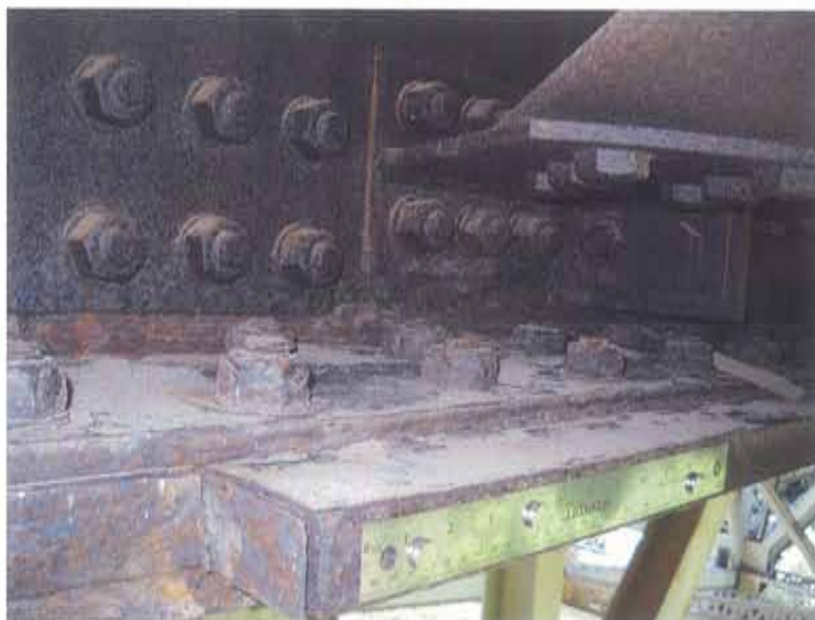
Photograph 87. Section loss in splice bolted connection components in lower flange of G3
