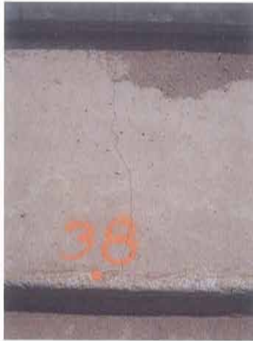
Photograph 25. Typical narrow to medium transverse cracking on sidewalk
