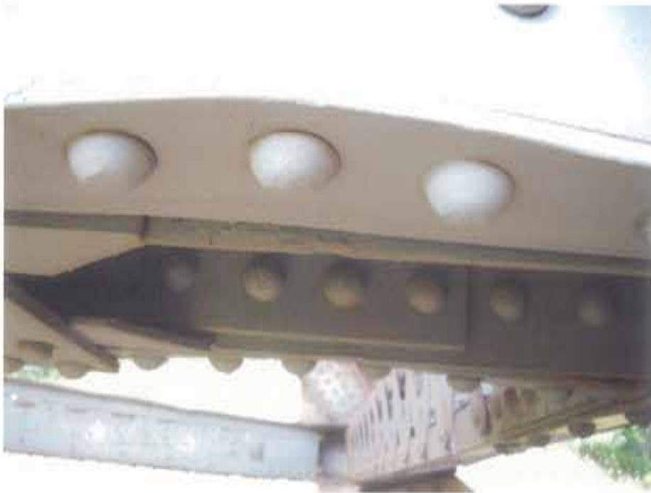
Photograph 72. Typical notch noted in distortions in lower chord flanges about west pier bearings
