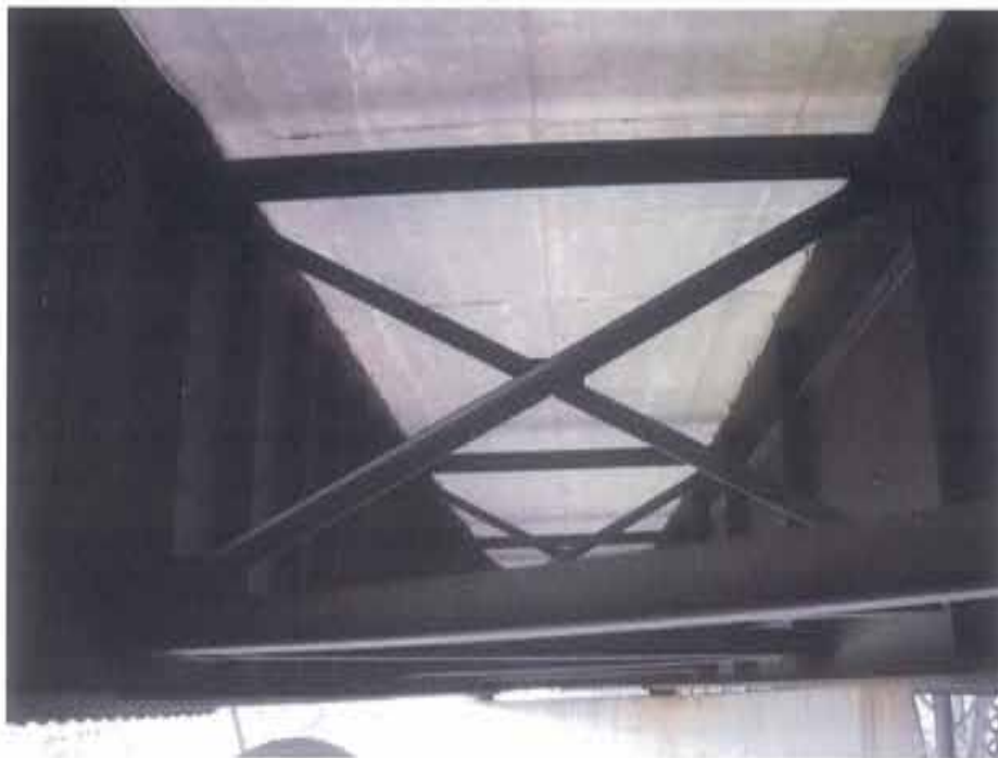
Photograph 42. Typical soffit condition of the north structure
