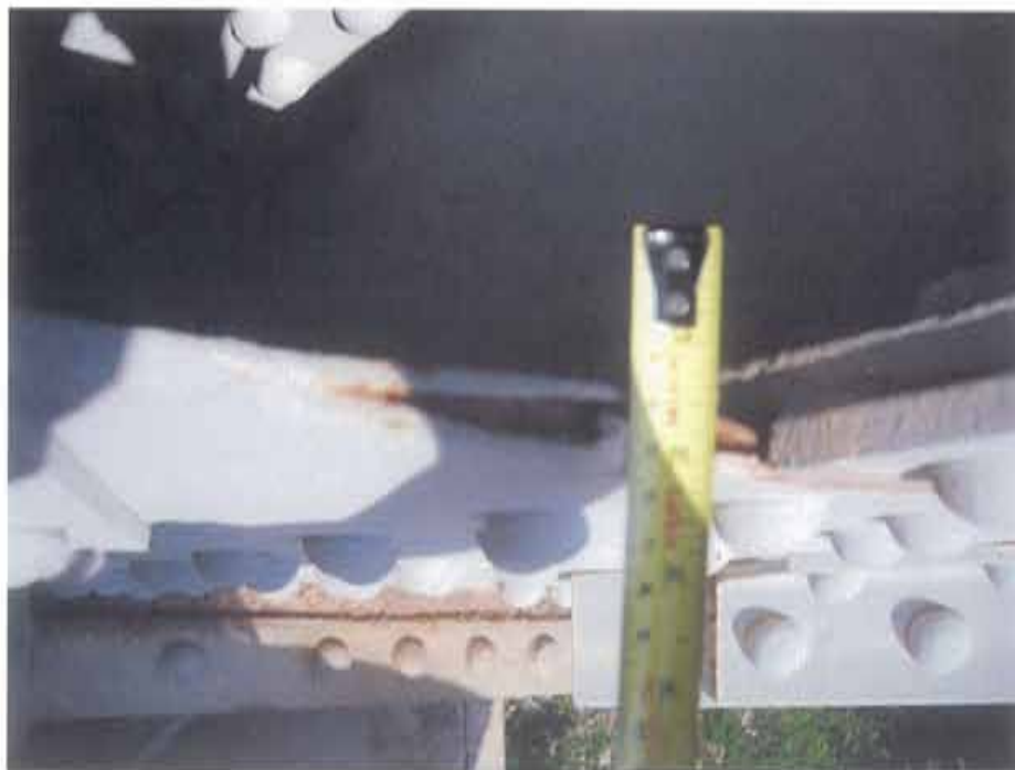
Photograph 60. Close-up of tear in south gusset plate at L12E
