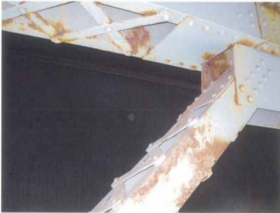
Photograph 45. Typical light corrosion noted on the upper chord member of truss T1
