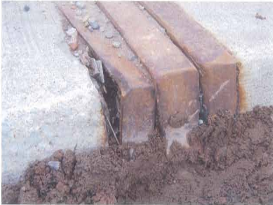
Photograph 15. Distortion of west sidewalk joint, facing south-west; note: impact damage on steel angle
