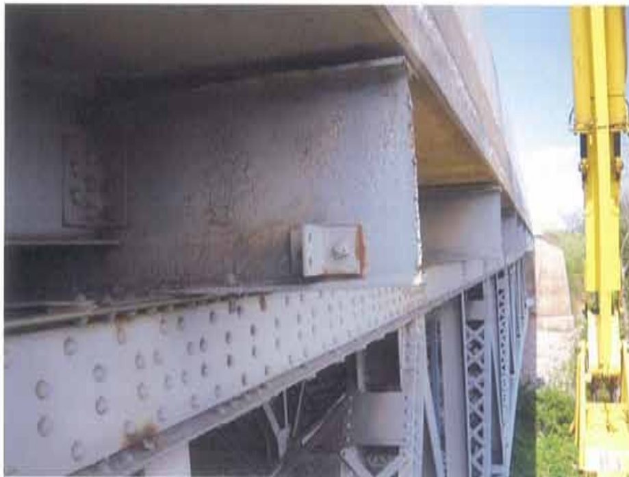
Photograph 40. South deck cantilever of south structure; note: delamination on top of transverse floor beam, and section loss of the transverse floor beam
