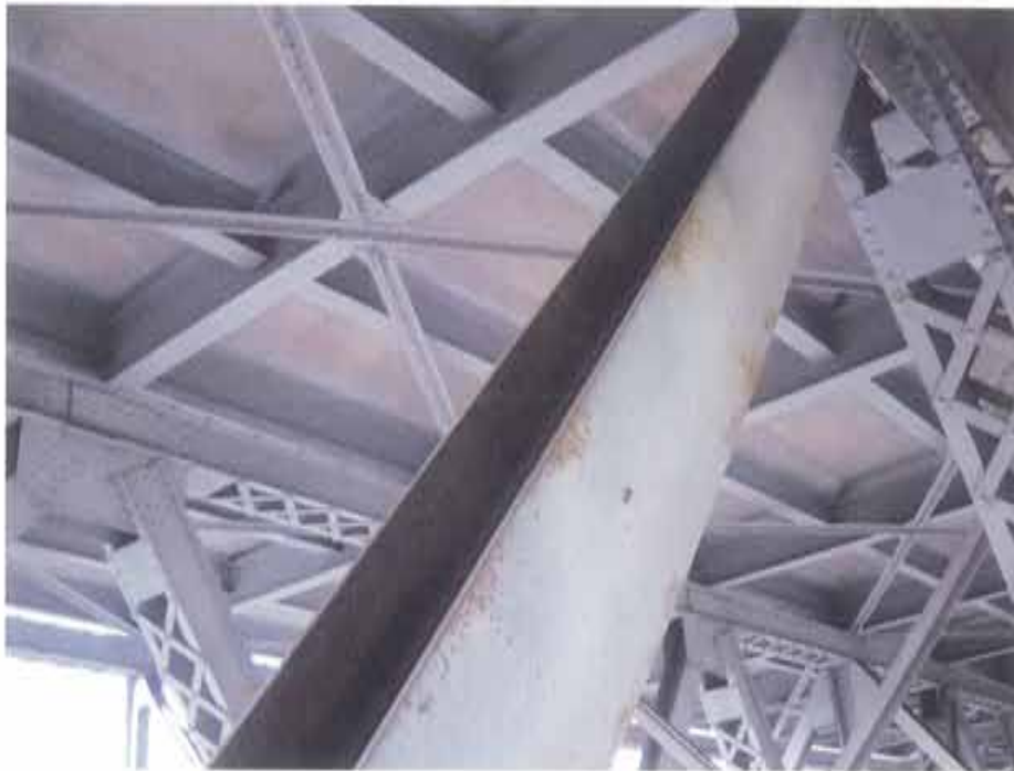
Photograph 61. Typical light corrosion noted in diagonal and vertical members of T1
