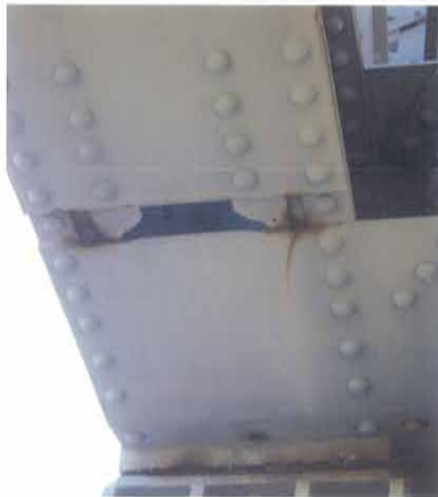
Photograph 58. Perforation in lower flange of T3/L28-L26E (10 mm)
