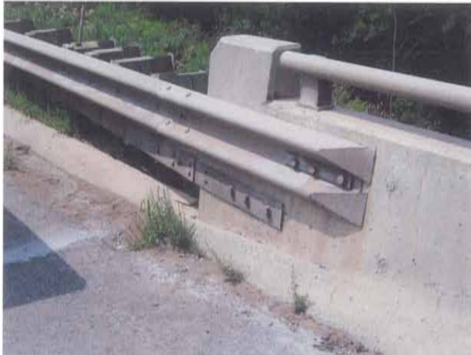
Photograph 30. Connection of steel beam guide rail to parapet wall at north west corner of bridge (typical)
