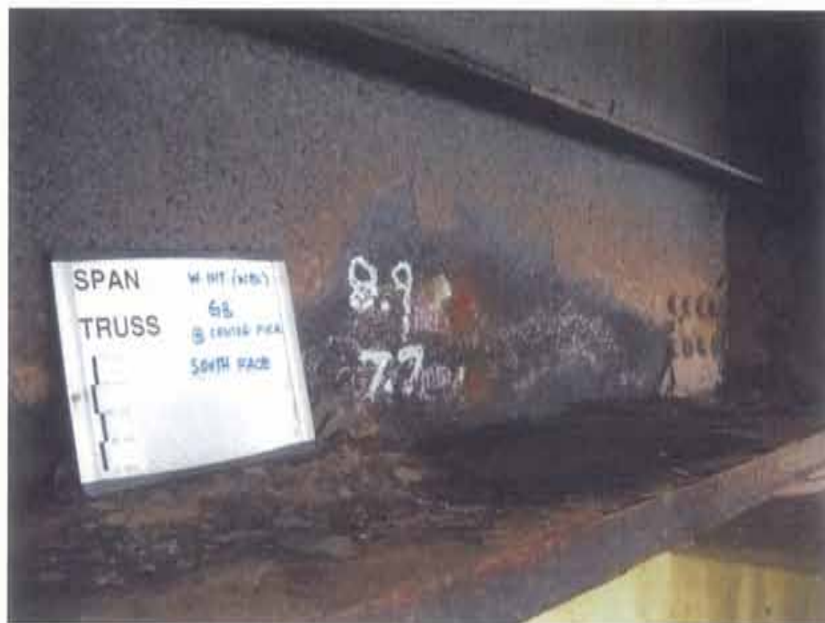
Photograph 84. Ultrasonic thickness measurements taken in areas of section loss; note: this photograph was taken in the same location as Photograph 83
