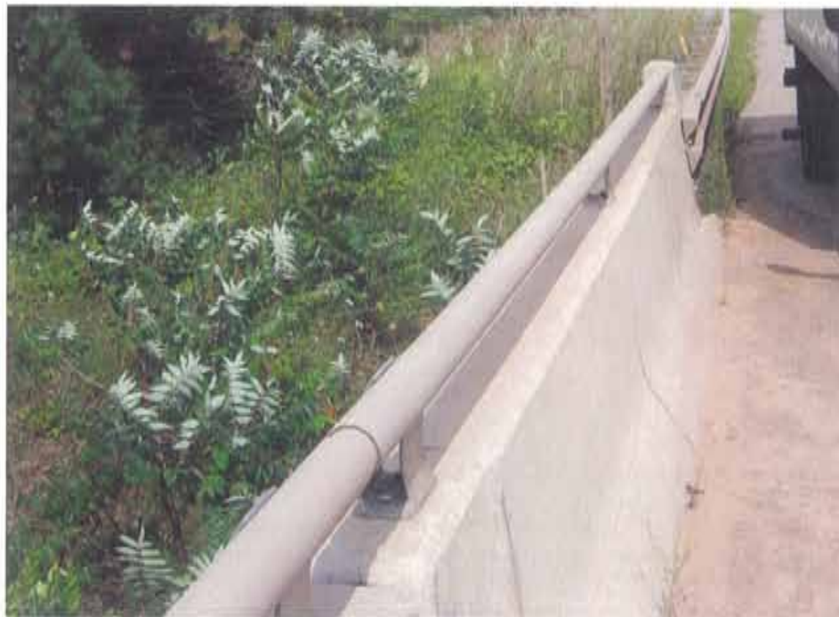
Photograph 24. Typical condition of railing; note: light surface corrosion
