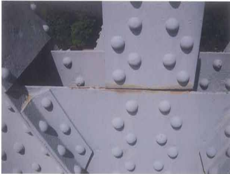
Photograph 59. Tear in south gusset plate of T3 at L12E
