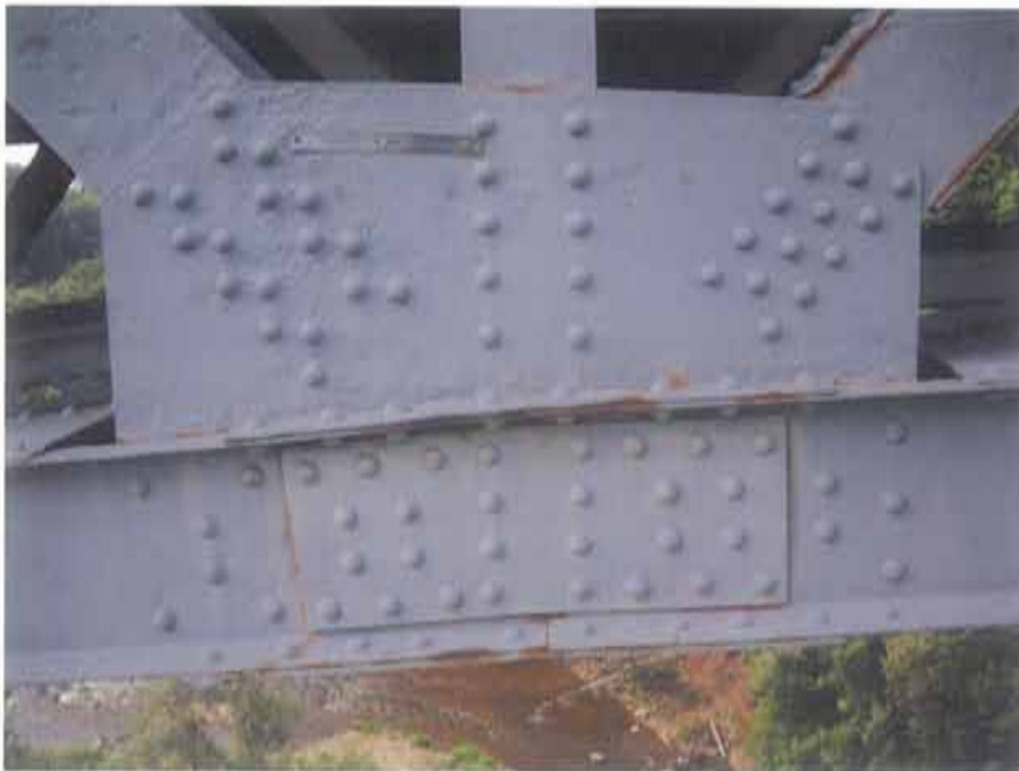
Photograph 54. Section loss due to previous and active corrosion, south gusset plate at T3/EL22 shown; note: ultrasonic thickness measurements taken to determine section loss
