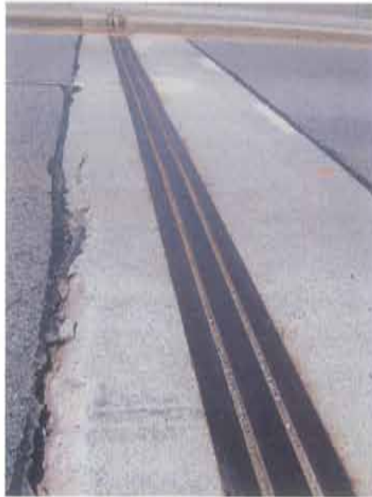
Photograph 13. Typical accumulation of debris within the transverse joints at the abutments; note: concrete disintegration at the concrete end dam (typical)
