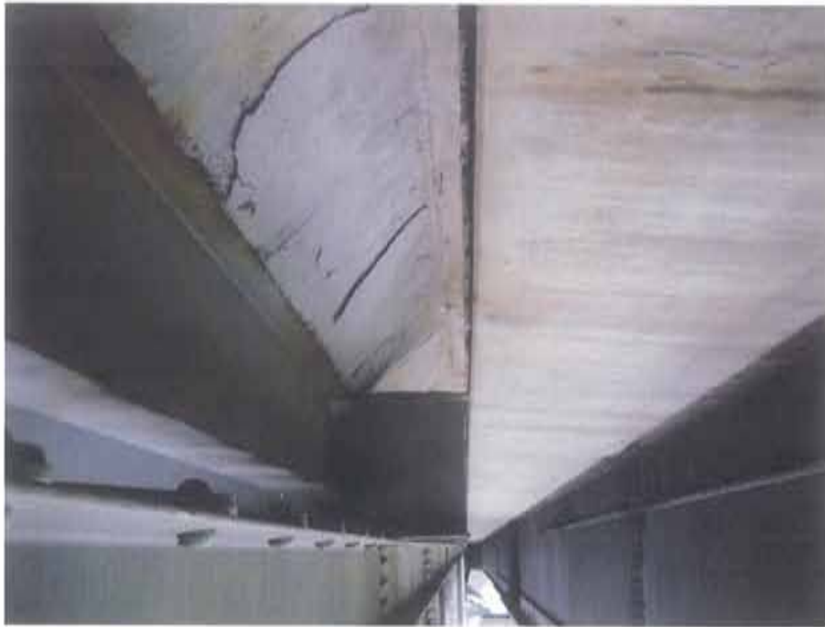
Photograph 39. Concrete delaminations in deck cantilever of south structure
