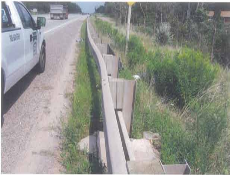
Photograph 31. Damage to south east steel beam guide rail
