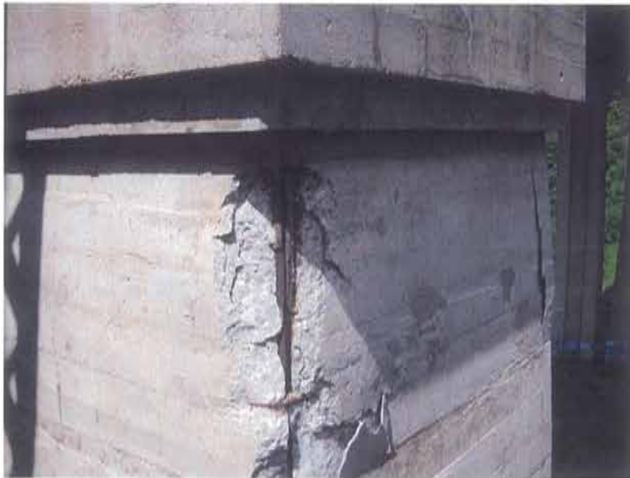
Photograph 67. Typical spalling and delaminations noted in the west pier of the south structure
