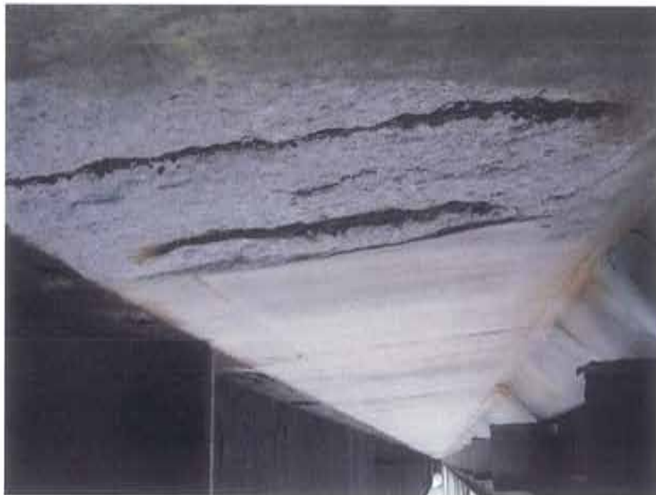
Photograph 10. Spalling in south deck cantilever of north bridge, looking east; note: photo shows the concrete deck cantilever at the centre median
