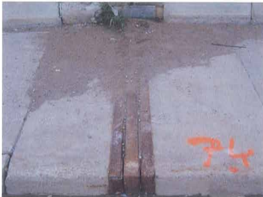
Photograph 12. Debris build-up in the east sidewalk joint of the south bridge; note: the large accumulation of debris build-up at this location may indicate the approach sidewalk has settled
