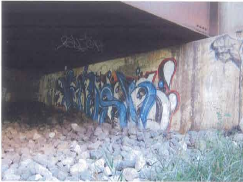
Photograph 17. Typical deterioration of abutment under north structure
