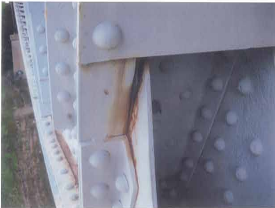
Photograph 52. Rust jacking noted in lower chord gusset plate
