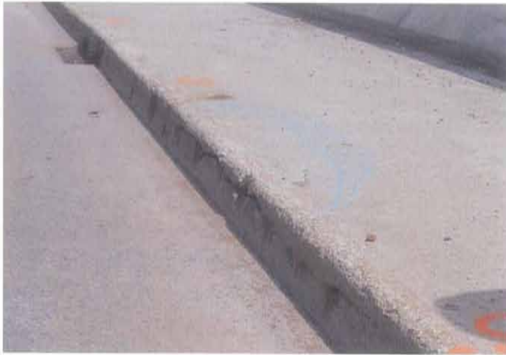
Photograph 27. Typical delamination in sidewalk
