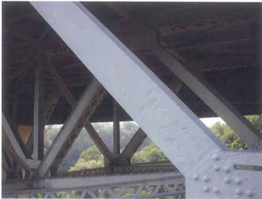
Photograph 63. Section loss due to previous corrosion in diagonal member T3/L22E-U23E
