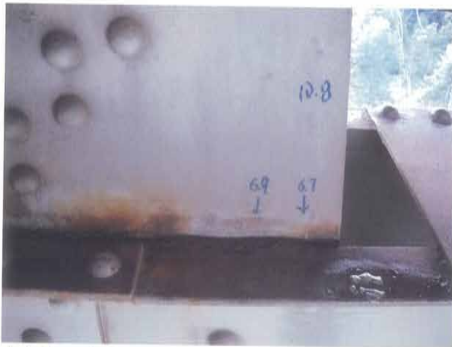
Photograph 50. Ultrasonic thickness measurements at T1/L12E (6.8 mm at section loss, 10.8 mm original thickness); see Photograph 49 for description
