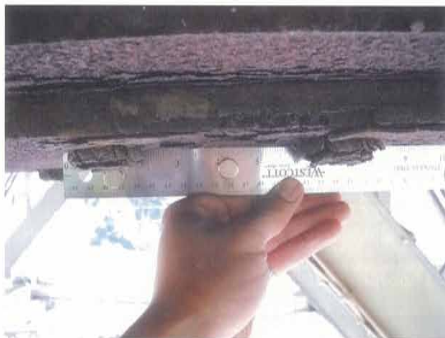
Photograph 88. Severe corrosion in splice bolted connection components of lower flange of G3
