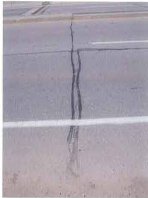
Photograph 29. Sealed transverse and longitudinal cracks at the east approach slabs (looking north)
