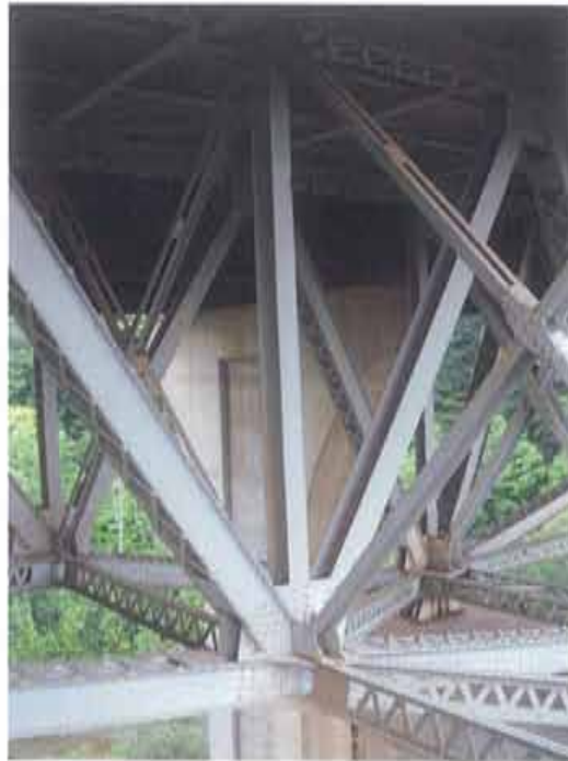
Photograph 73. Typical condition of T2 condition, T2/L26W shown
