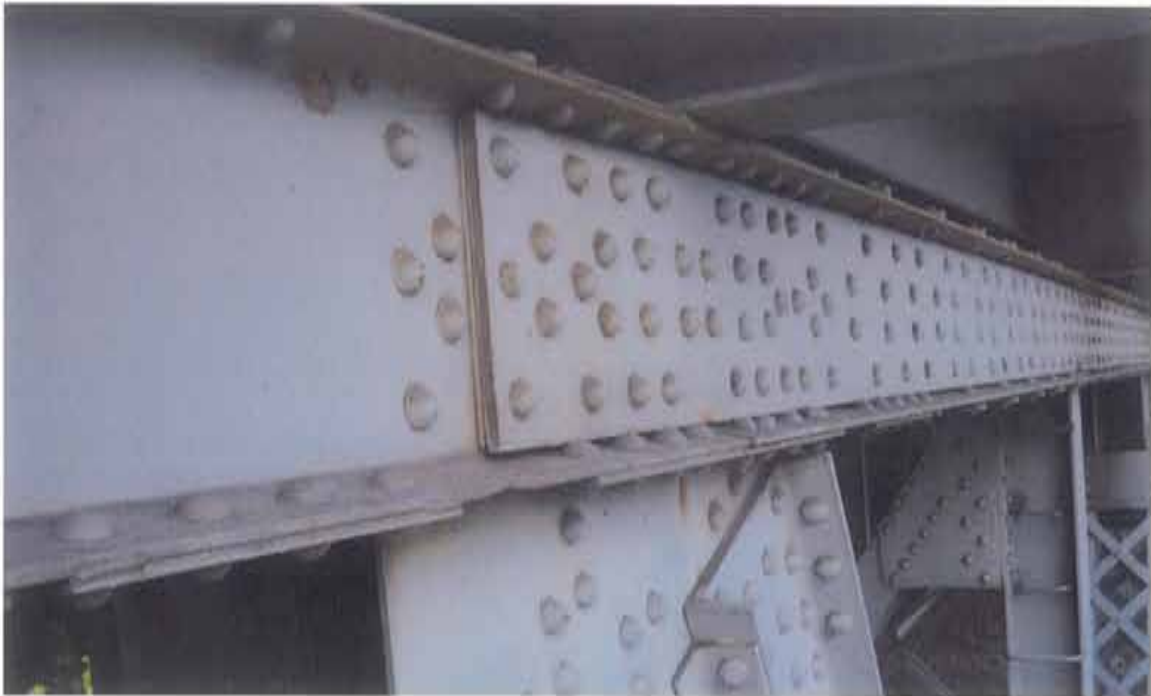
Photograph 47. Typical condition of the upper chord members of truss T3
