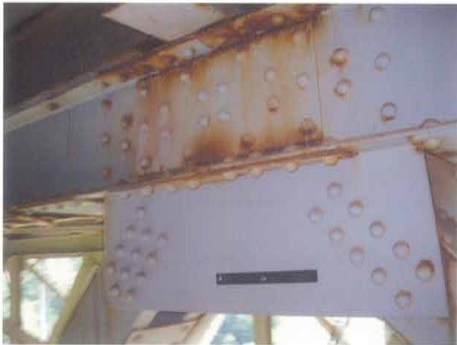
Photograph 46. Typical light corrosion noted on the upper chord member of truss T1
