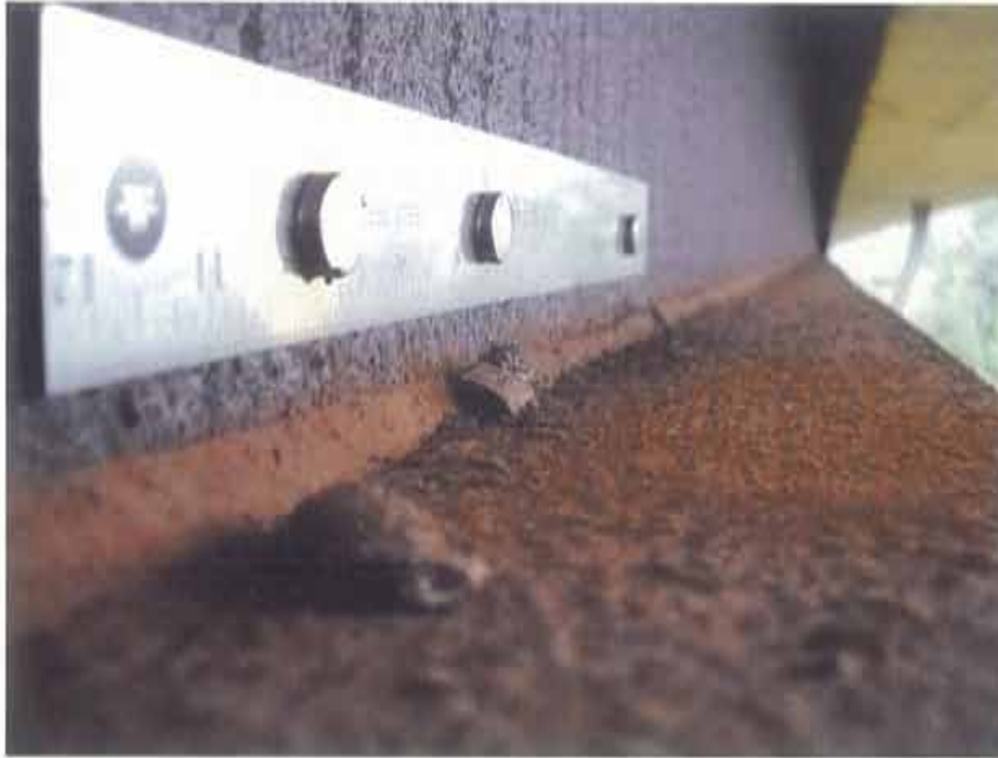
Photograph 81. Longitudinal web stiffener plate weld broken at several locations, G1 shown
