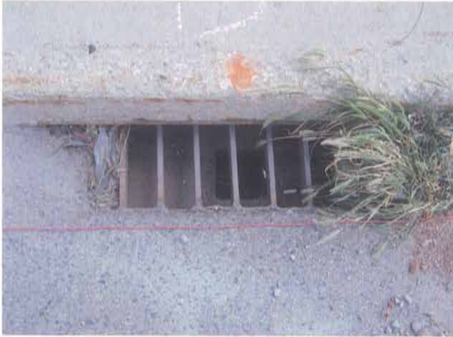
Photograph 19. Typical deck drain with vegetation growth
