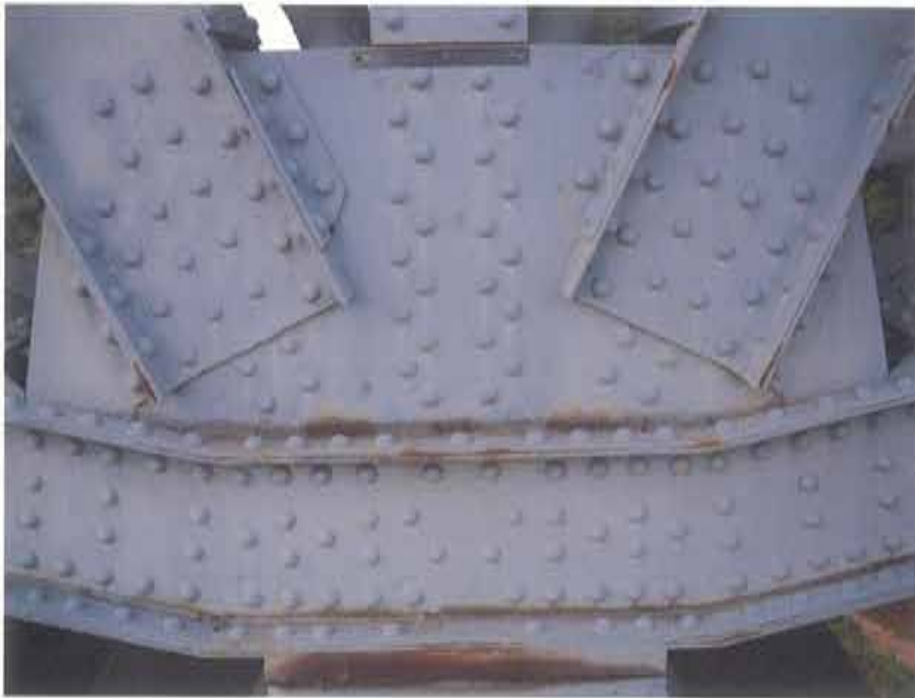
Photograph 53. Section loss due to previous and active corrosion, south gusset plate at T3/L28 shown; note: ultrasonic thickness measurements taken to determine section loss
