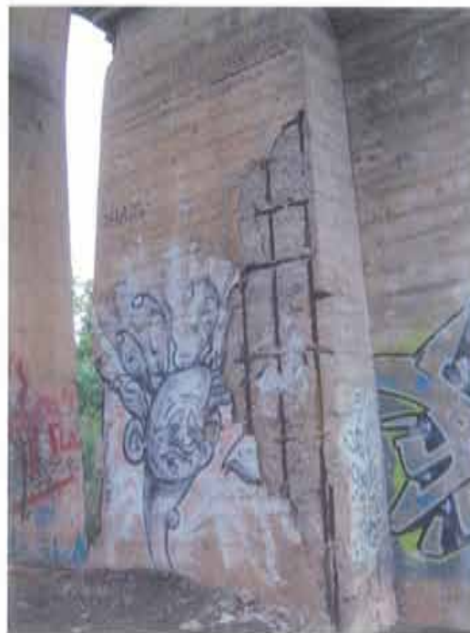
Photograph 68. Large concrete spalling in west face of west pier
