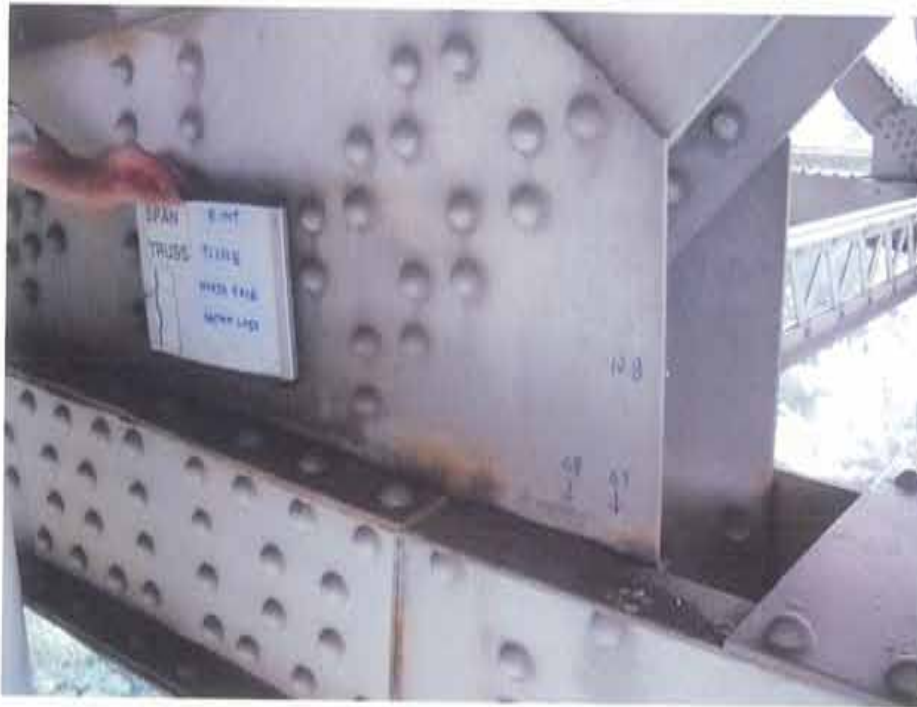
Photograph 49. Section loss in lower chord gusset plate at T1/L12E due to seam corrosion
