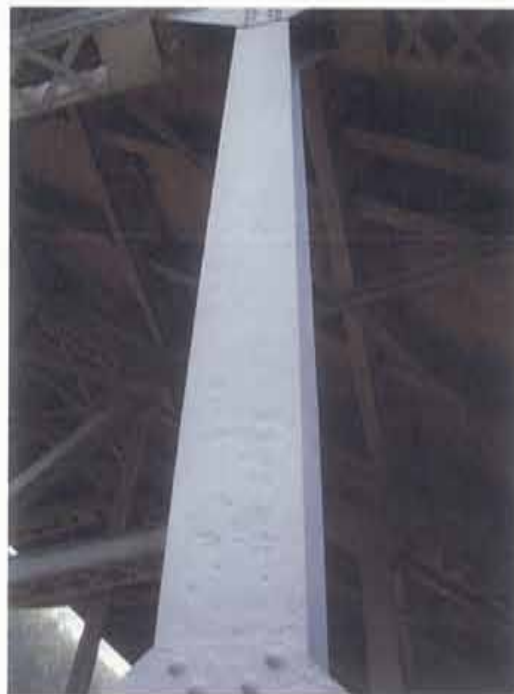
Photograph 64. Section loss due to previous corrosion in vertical member T3/L22E-U22E
