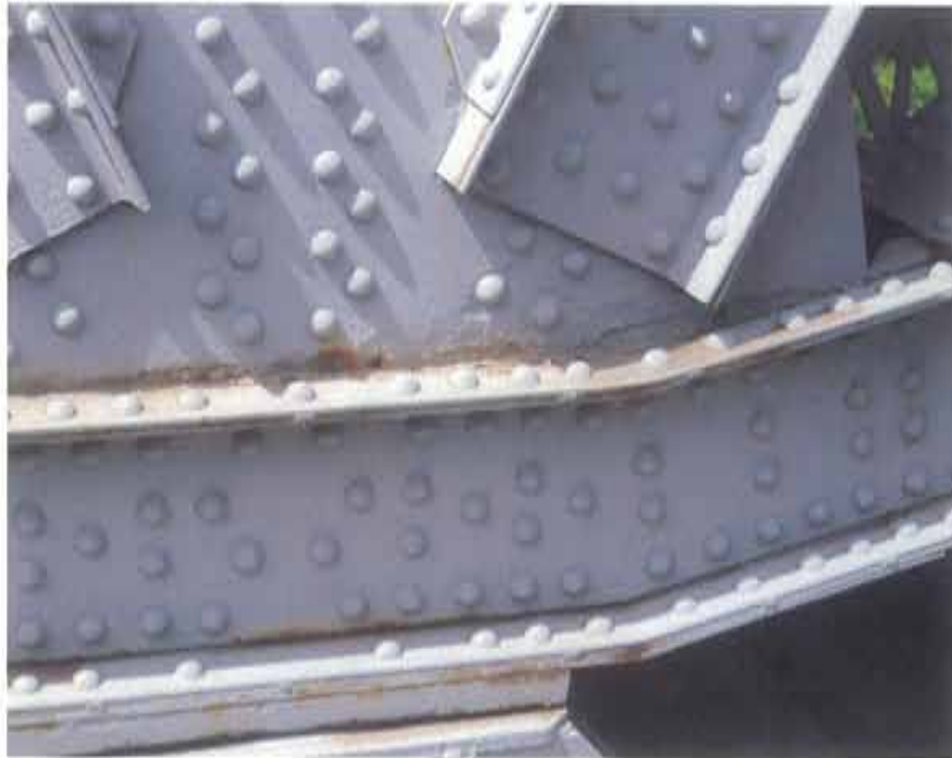
Photograph 57. Perforation in south gusset plate of T3/L12W (12 mm diameter)
