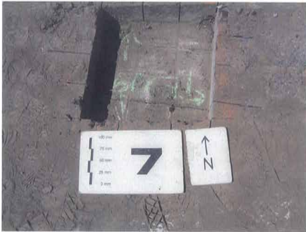
Sawn Asphalt S7
