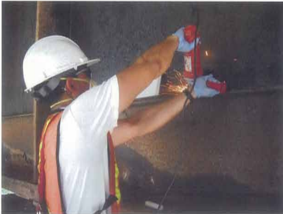
Photograph 82. Metal grinder used to clean surface prior to testing of section loss, G3 shown
