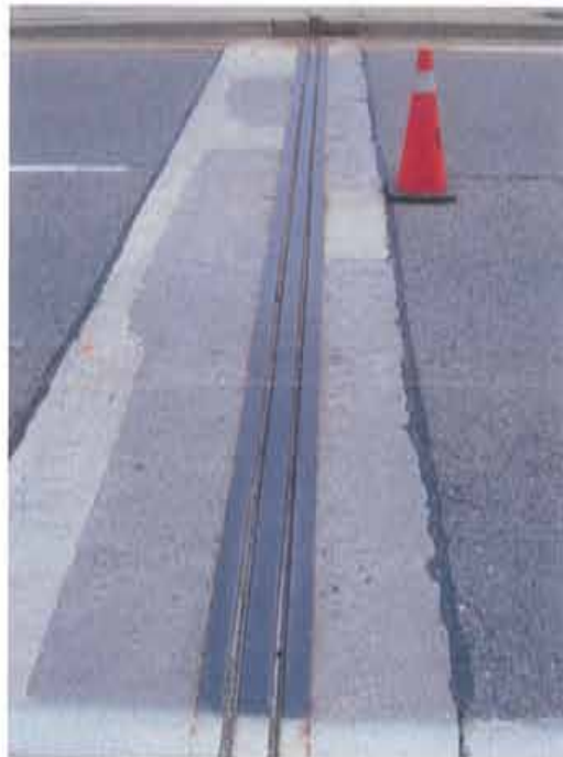
Photograph 14. Typical condition of concrete patching in concrete end dams and ballast wall (completed during the 2004 rehabilitation work)
