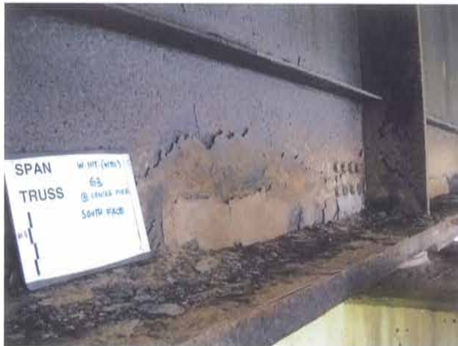
Photograph 83. Typical rust expansion noted in web plate of G3
