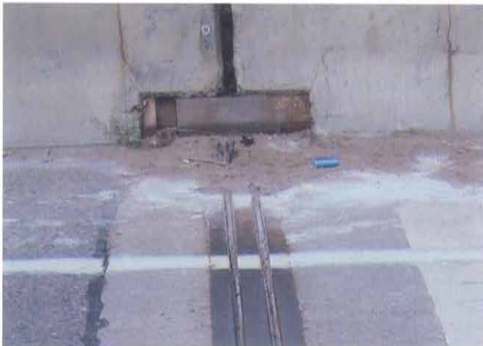
Photograph 16. Pop-out of joint seal at the west joint of the north structure, looking north; note: pop-out is typical of the ends of all the joints on the north structure
