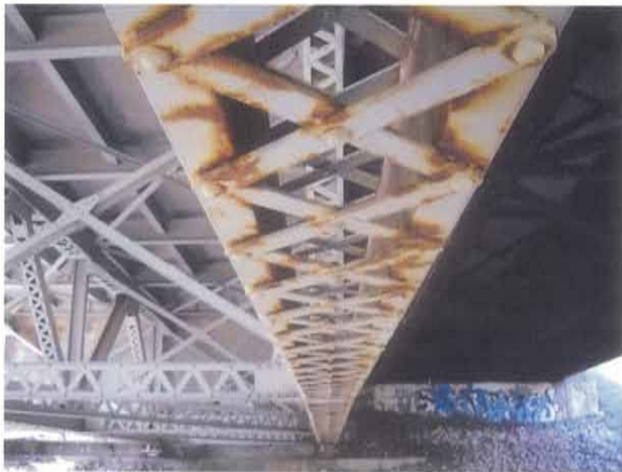
Photograph 48. Typical light corrosion noted on the lower chord members of truss T1
