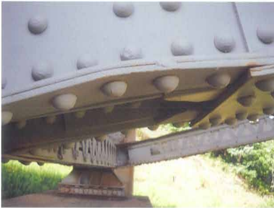
Photograph 71. Distortion in T2/L12W-T2/L14W about west pier bearings
