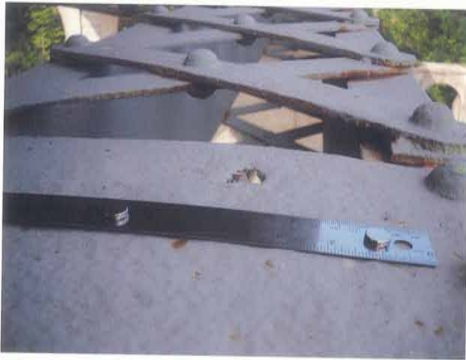
Photograph 55. Perforation in upper batten plate of T3/L22E-L20E (20 mm diameter)
