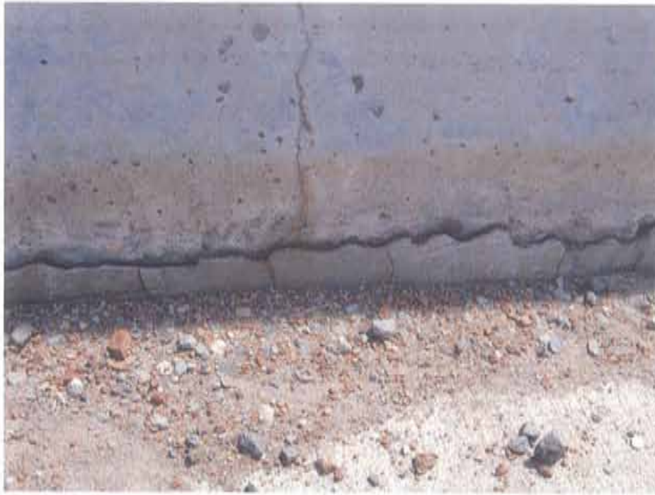
Photograph 23. Concrete disintegration at the base of the south barrier wall
