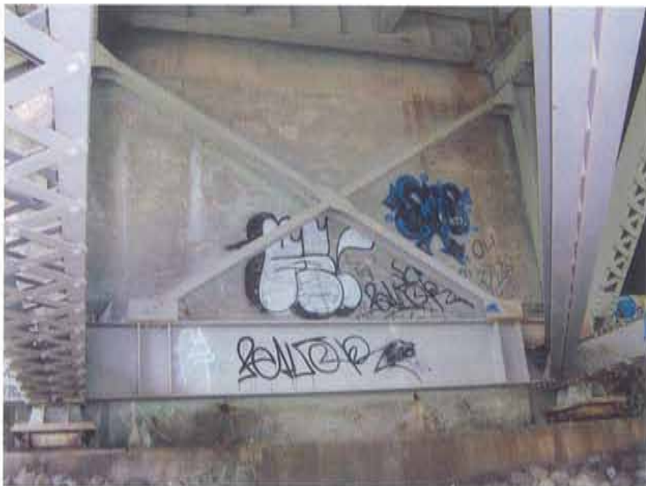
Photograph 18. Typical deterioration of abutment under south structure
