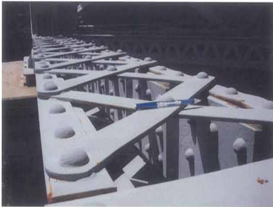
Photograph 51. Light seam corrosion noted in lower chord members of T3
