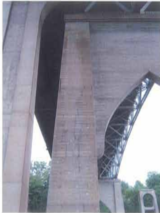
Photograph 69. Centre pier contained areas of vertical narrow concrete cracking
