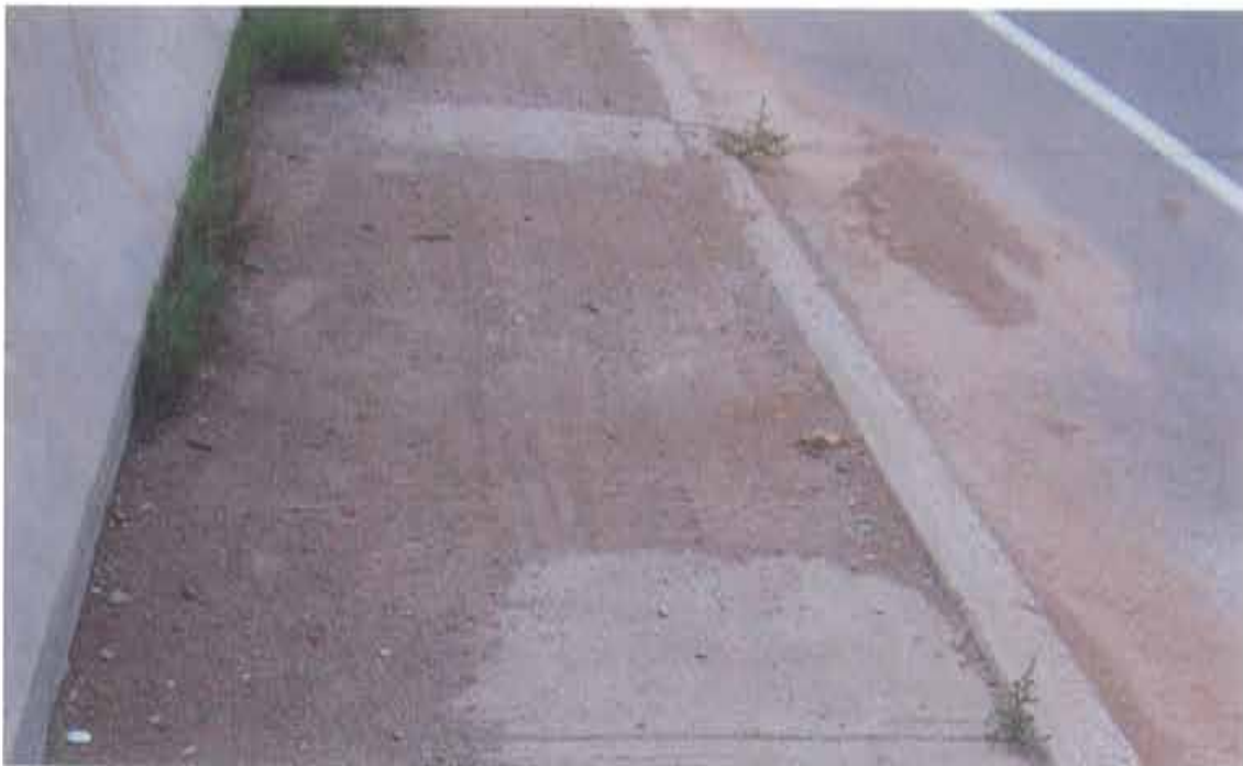
Photograph 28. Typical settlement of the sidewalk and accumulation of debris (located near the abutments)
