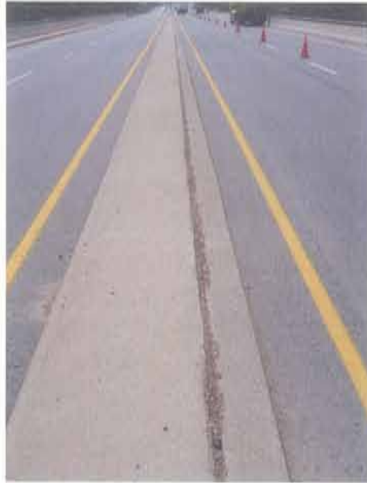
Photograph 9. Typical condition of centre longitudinal joint, looking west
