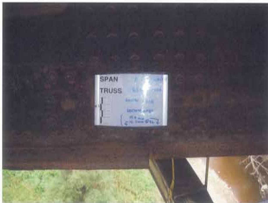
Photograph 86. Section loss in bolt heads at splice plate and section loss in lower flange, G3 shown
