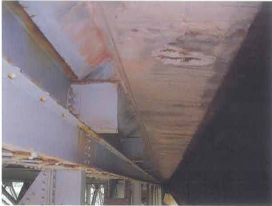
Photograph 11. Typical deterioration of deck cantilever at the centre median, looking west; note: spalling, rust staining, wet staining and transverse cracking
