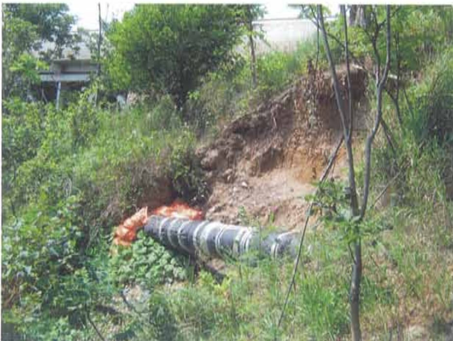
Photograph 38. Exposed pipeline to the southeast of the bridge
