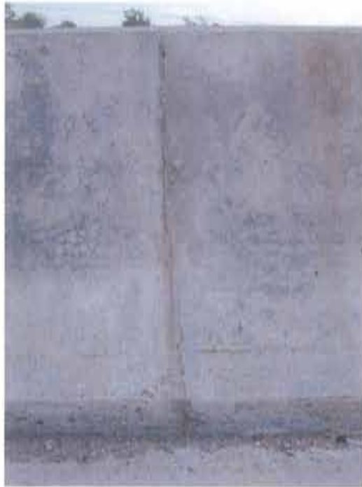
Photograph 21. Typical vertical cracking with staining on barrier wall
