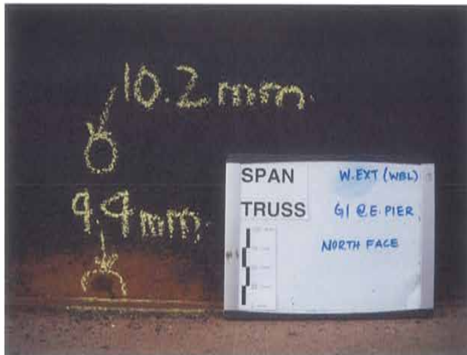
Photograph 85. Nominal section loss in web plate of G1
