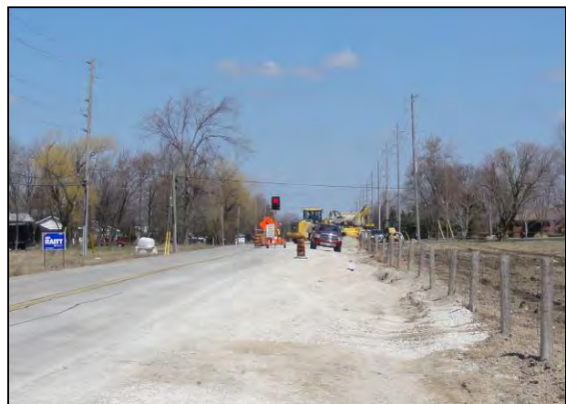
Plate 2: Looking east along Britannia Road at the construction activity west of Sixth Line.
