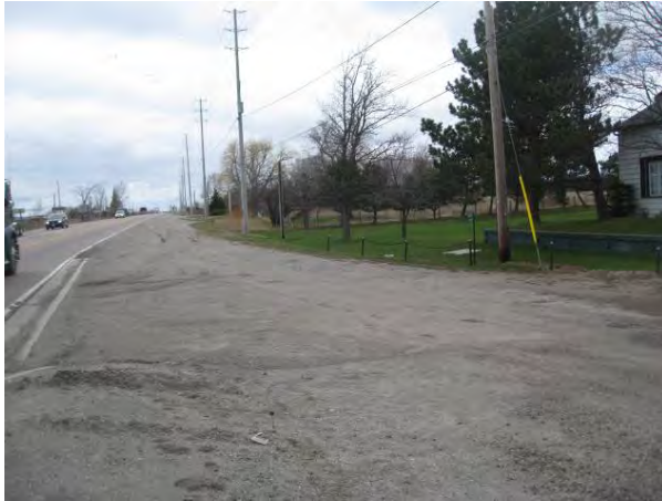
Plate 7: Northwest view up RR 25. Disturbed on both sides between ROW. Potential beyond ROW on right.
