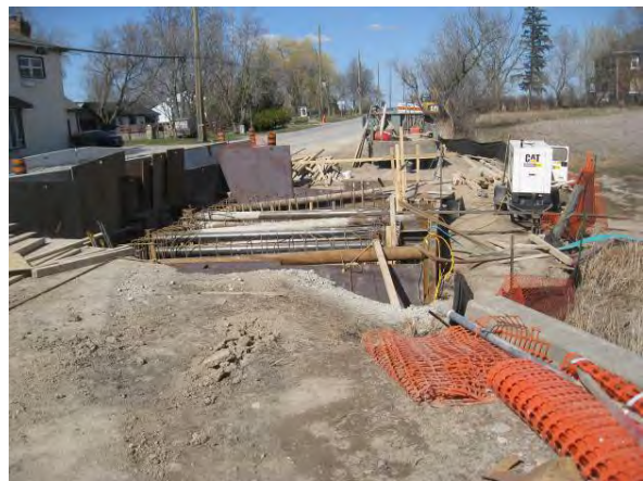
Plate 24: Northeast view of bridge reconstruction of intersection at Britannia Rd and Fourth Line. Disturbed with no potential.
