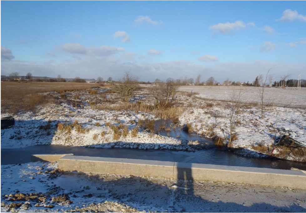
Updated Photos for Crossing 6, taken January 20, 2013 (upper left) - looking upstream (lower left) - looking downstream (lower right) - looking at upstream culvert face
