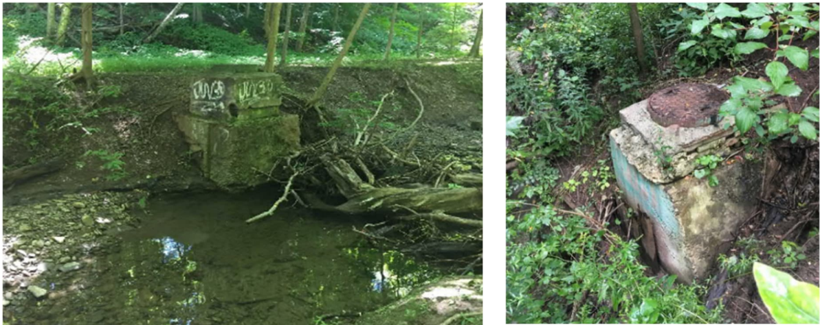
Figure 4-2: Exposed Maintenance Holes in Creek Corridor
